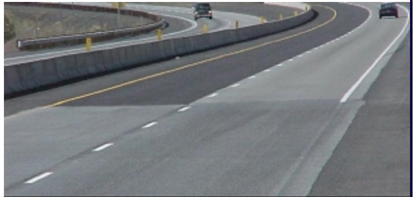
Durables vs. paint: The project at the top used all inlaid durable striping. Below, solvent-based paint was used, but the centerline was an inlaid durable. Both projects are about 8 months old; the bottom edge lines were painted with regular paint only a few months prior to this picture.
