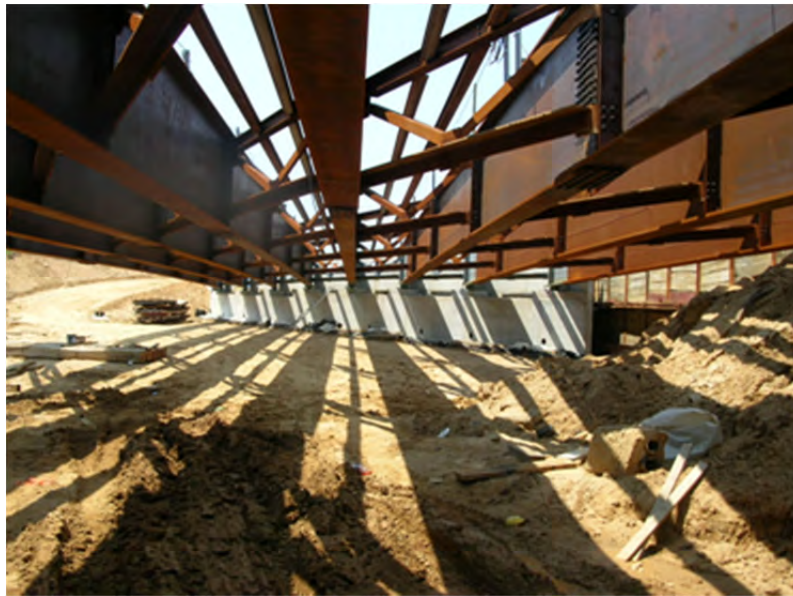
Figure 1.5: Churchman Road Bridge Delaware skewed intermediate cross-frames
