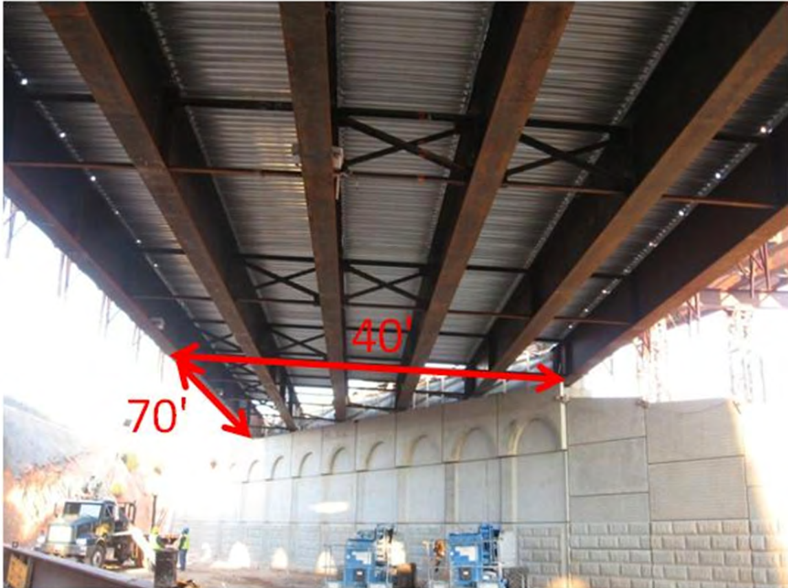
Figure 1.3: Skewed bridge support offset
