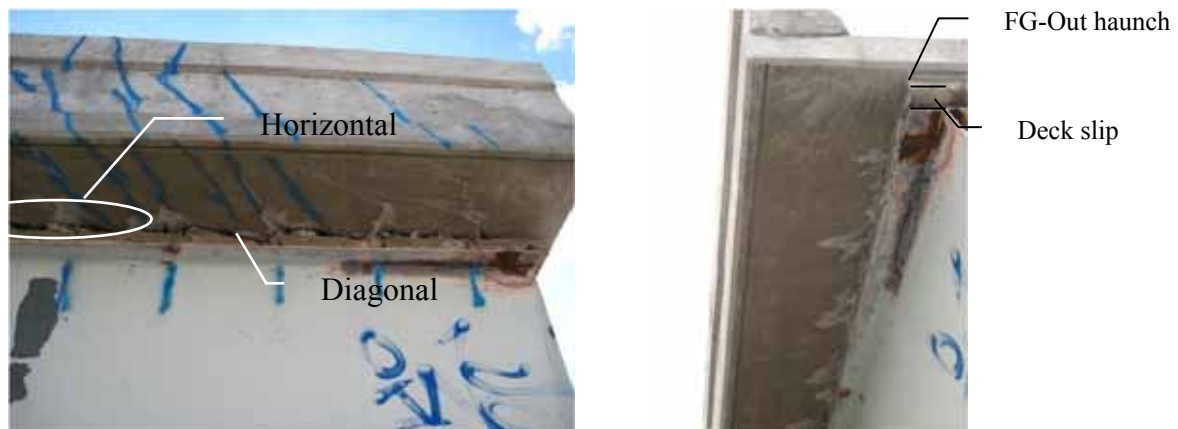
Figure 5.28: Slip between the deck and girder top flange along FG-Out
