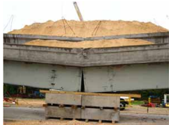
(b) Collapsed bridge
