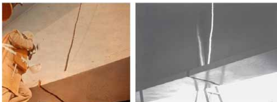
Figure 1.2: Opposing views of the Neville Island Bridge girder fracture
