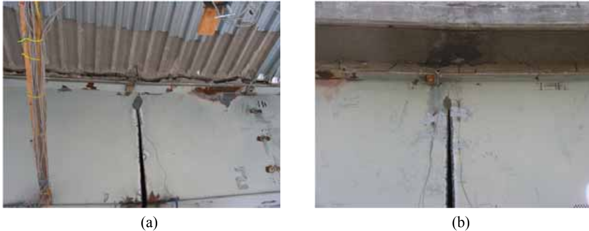
Figure 5.12: Haunch separation of fractured girder
