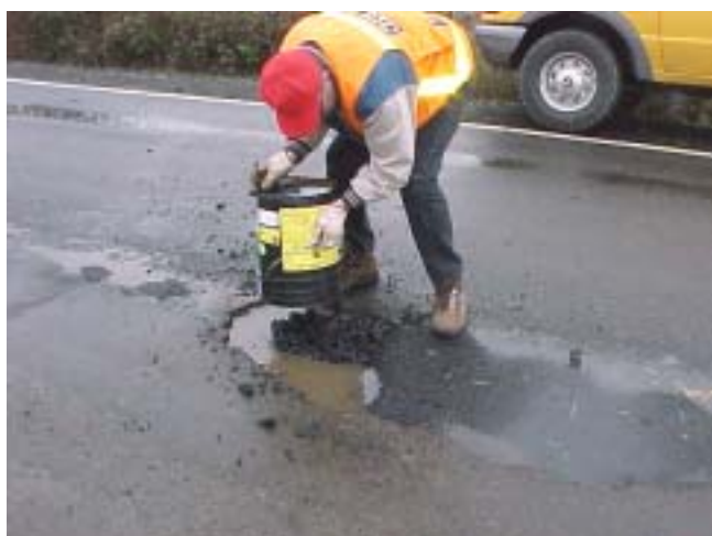
A maintenance worker fills a pothole on Century Drive in Albany with TAG 8000 mix
