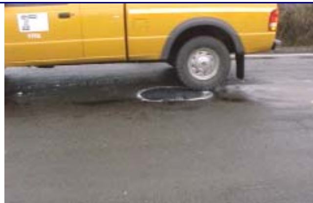
A pickup truck drives over the filled pothole for compaction of the mix
