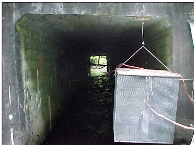
Upstream end of the culvert on Big Noise Creek, Oregon where the short-term controlled release study was performed. The wire cage is the upstream fish trap for fish that swim out of the culvert.
