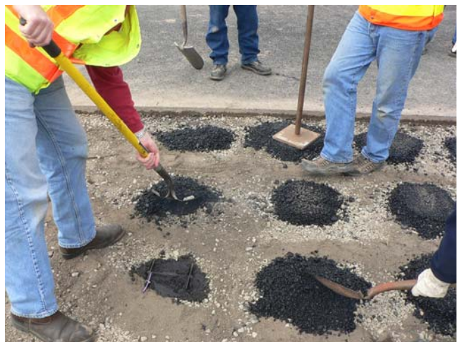
Placement of asphalt over the strain gages with light compaction to minimize gage movement during the paving
