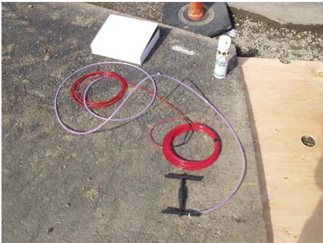
Strain gage with protective nylon sheath installed on the first 12 ft of the lead-in wire
