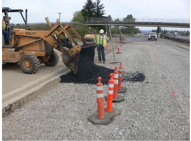
Additional asphalt being placed over the gages prior to paving over the rubblized concrete base
