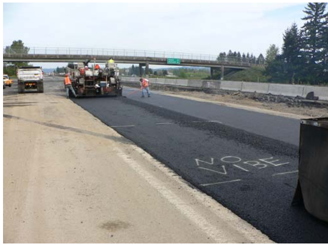
After the first lift of asphalt over the rubblized concrete base. Notice that vibratory rollers were not used over the gages.
