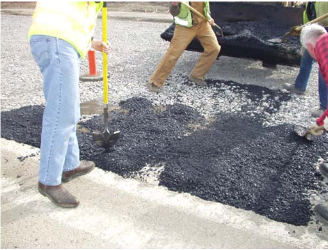
Placement of asphalt over the strain gages to minimize movement during paving over the rubblized concrete base
