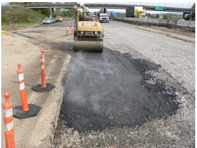
Initial compaction of the asphalt over the strain gages prior to paving over the rubblized concrete base
