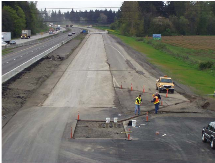
Overlooking the instrumentation site in the southbound lane of I-5 at milepost 239
