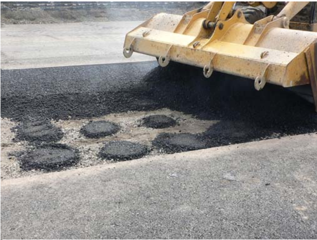
Completing the trench fill of asphalt over the strain gages on the aggregate base
