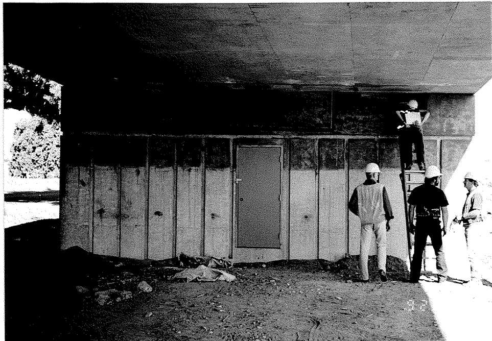
Figure 3.4 Access to strong motion instrumentation is located under the North end of BR# 9669A.
