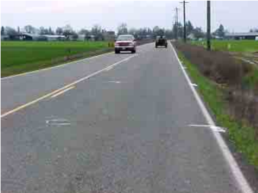
Figure 4.4: Wallace Road manufactured potholes, looking south
