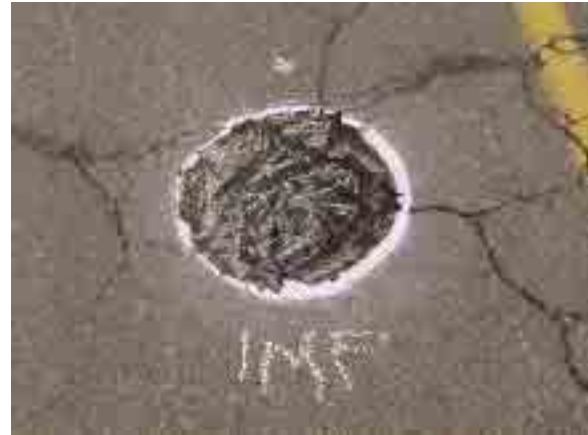
Figure 4.2: Manufactured pothole at Century Drive
