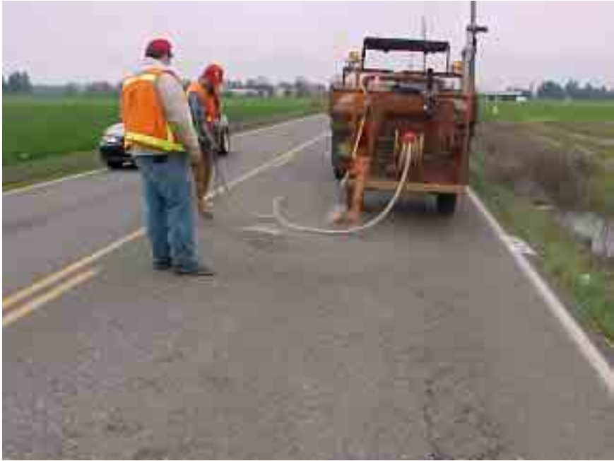
Figure 4.3: Wallace Road pothole manufacturing
