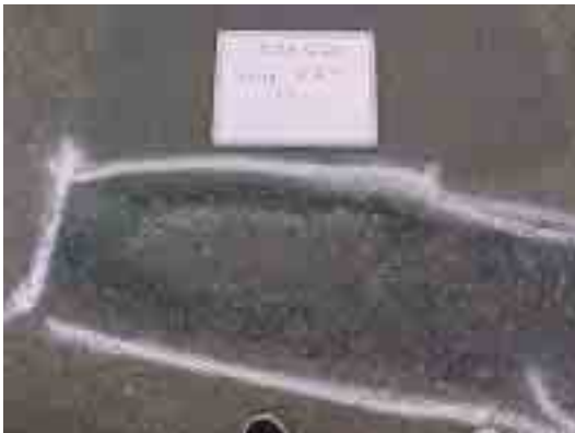
Figure B.4: Close-up of Perma Patch failure
