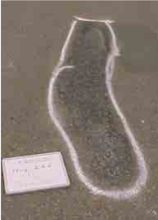
Figure B.3: Perma Patch failure on Hwy 226
