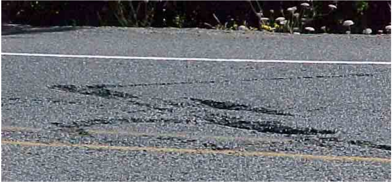
Figure B.1: Hwy101 at Ona Beach State Park prior to patching
