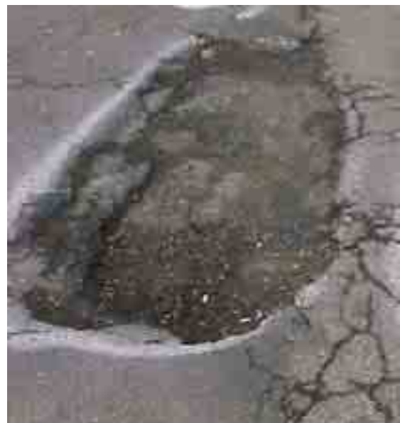
Figure 4.10: Albany Mix complete failure
