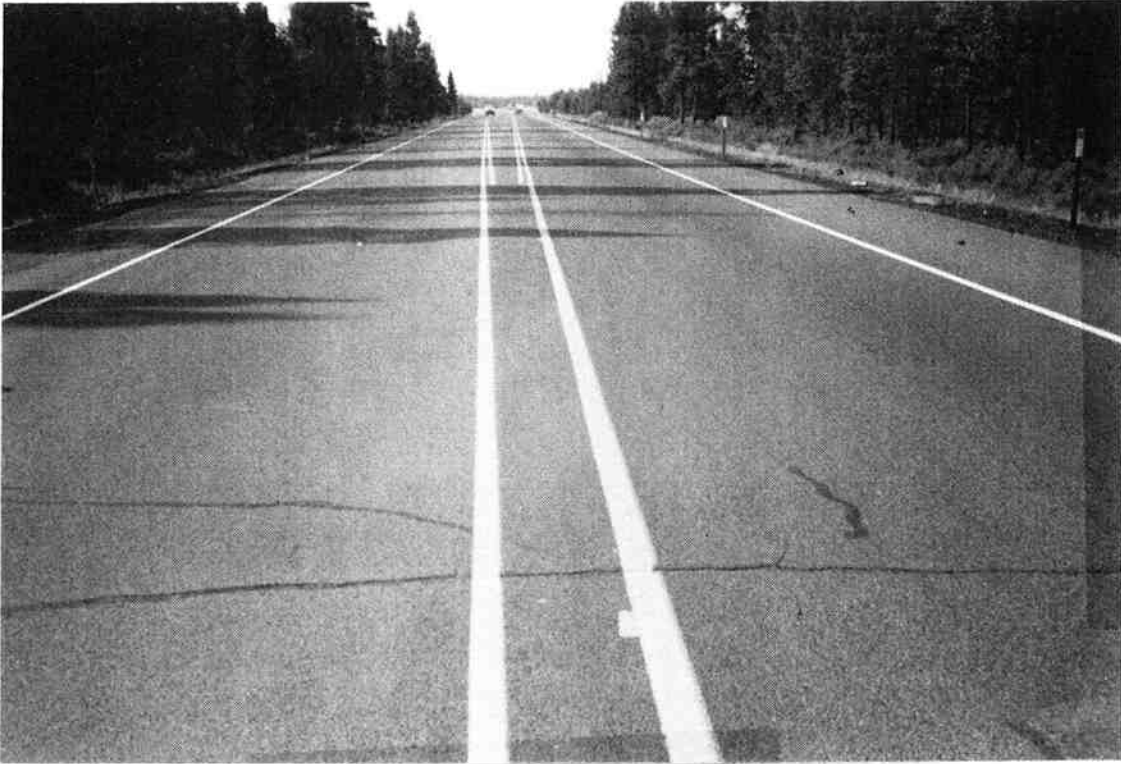
(a) Typical transverse crack in overlay during 1989. Crack has been covered with sealer.
