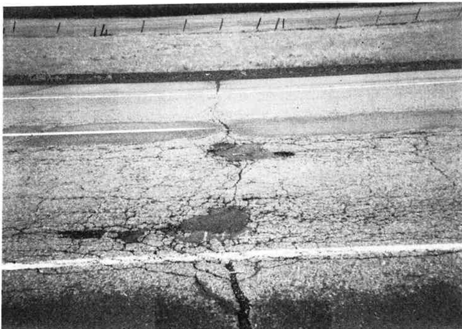
(b) Typical transverse crack in pavement before construction.
