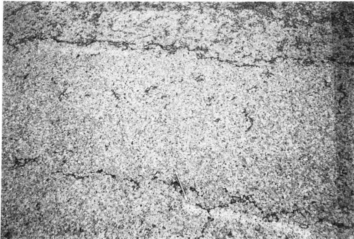
(b) Cracking and ravelling typical of 6% of wheeltrack length. Pits and cracks have retained moisture and appear as dark areas.
