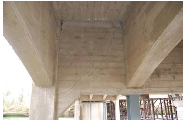
Bent cap with highlighted crack
