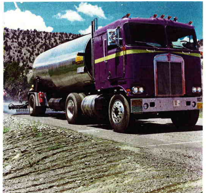
d. Close-Up of Distributor
