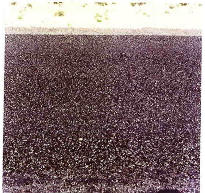
h. Final Surface
