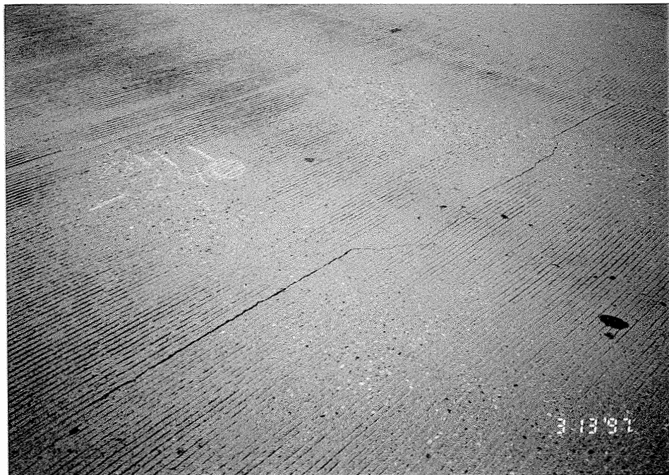
Figure 5.3 Bridge #1417N, minor cracking is rare.
