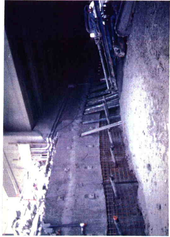
Drilling and placing temporary casings at nail locations; Dywidag bars were later inserted and the boreholes pressure grouted prior to placing the shotcrete application.
