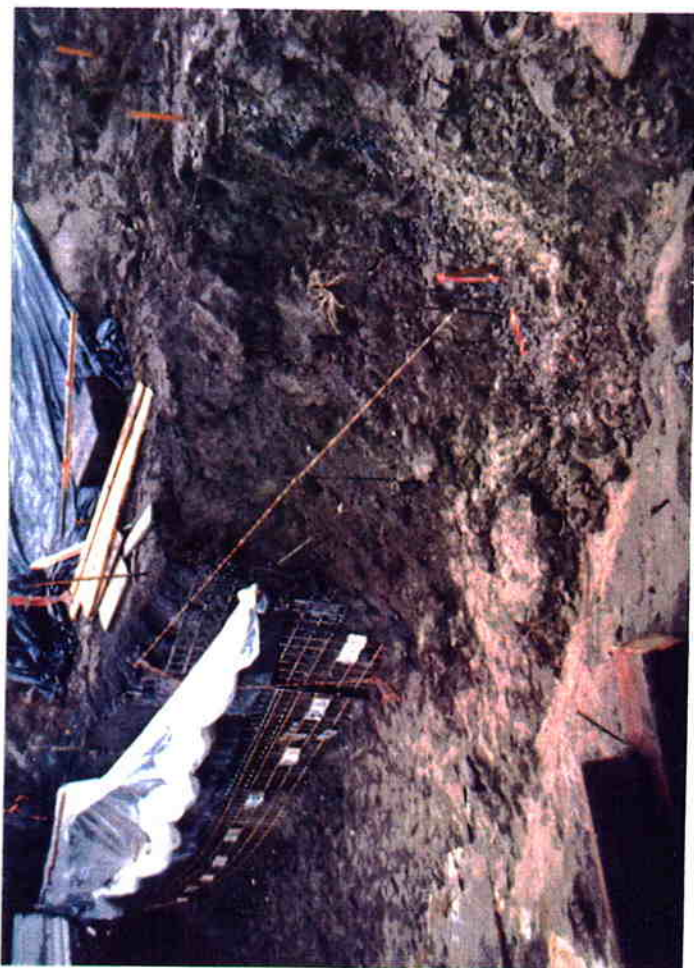
The westerly most 12-foot wall segment collapsed overnight due to over- excavation.
