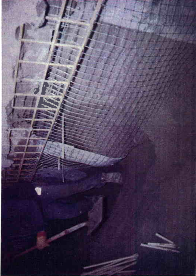
Soil sloughing at the open face during the placement of the chicken wire mesh.
