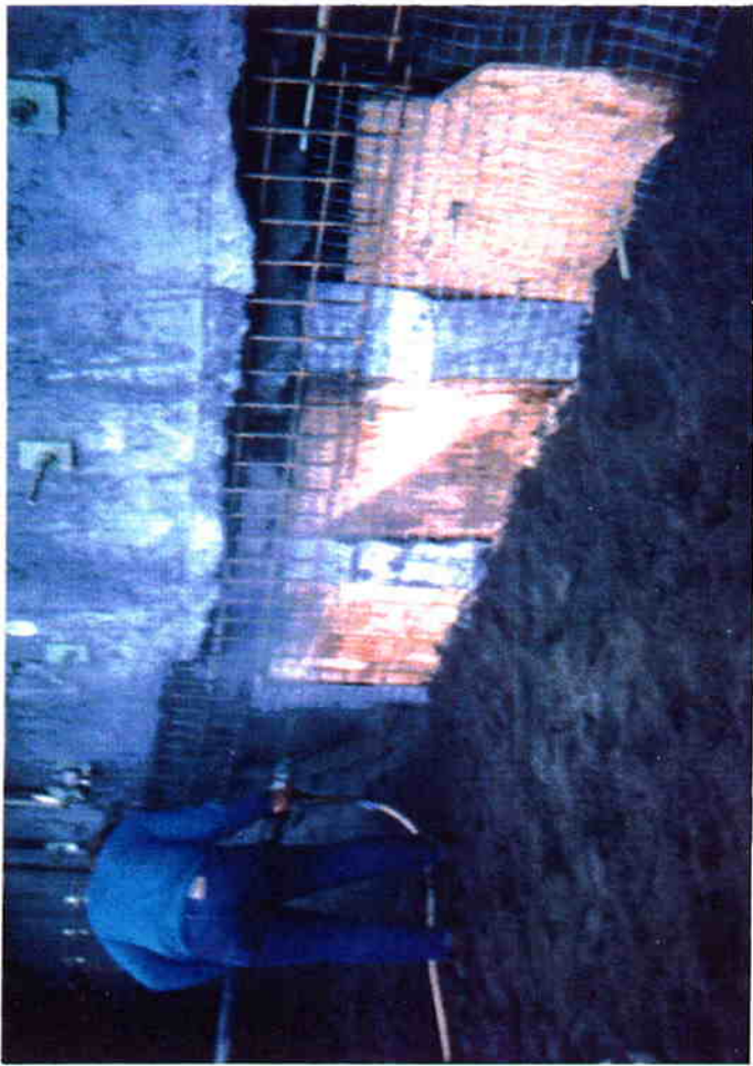
Collapsed face was formed with plywood and shotcrete was placed behind the forms to replace the sloughed material.
