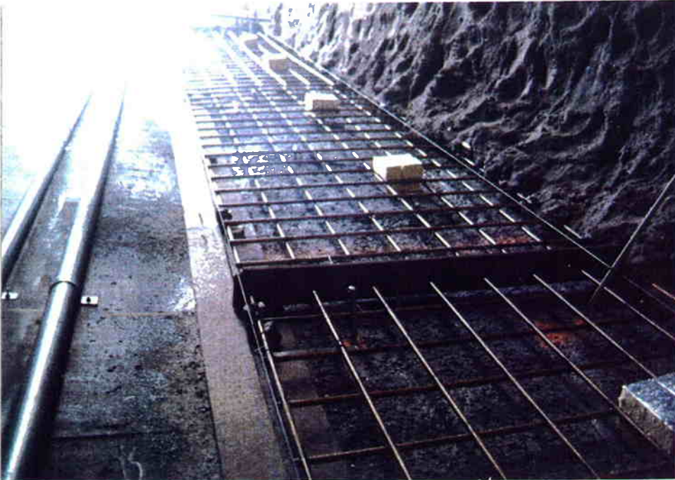
Steel welded wire mesh reinforcement corresponding to first shotcrete application. Notice (1) blockouts at nail locations; (2) preformed expansion joint filler at the expansion joint location; and (3) stretched piano wires to control face thickness during shotcrete placement.
