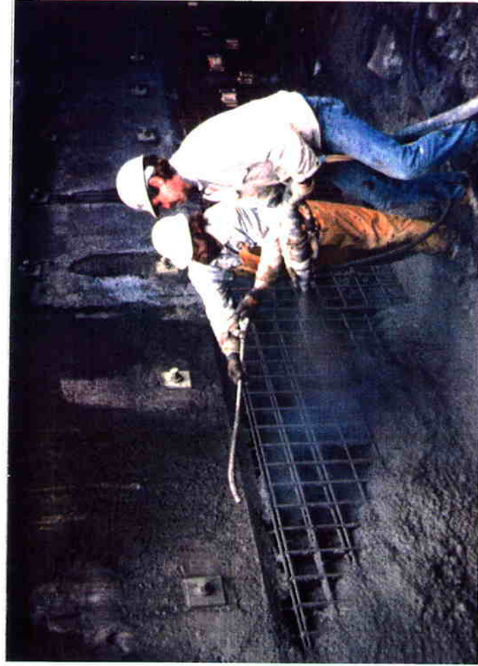
Mozzleman placing first structural shotcrete application; helper with an air blow pipe keeping work area free of rebound material.
