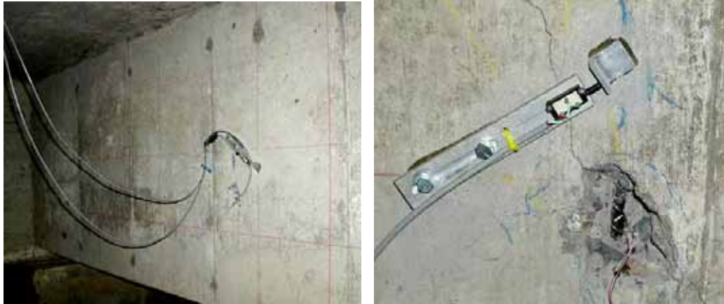
Figure 9.2: Example instrumented location of stirrup crossing diagonal crack
