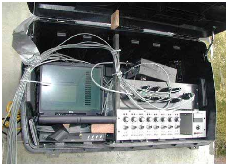
Figure 9.3: Instrumentation enclosure on pier
