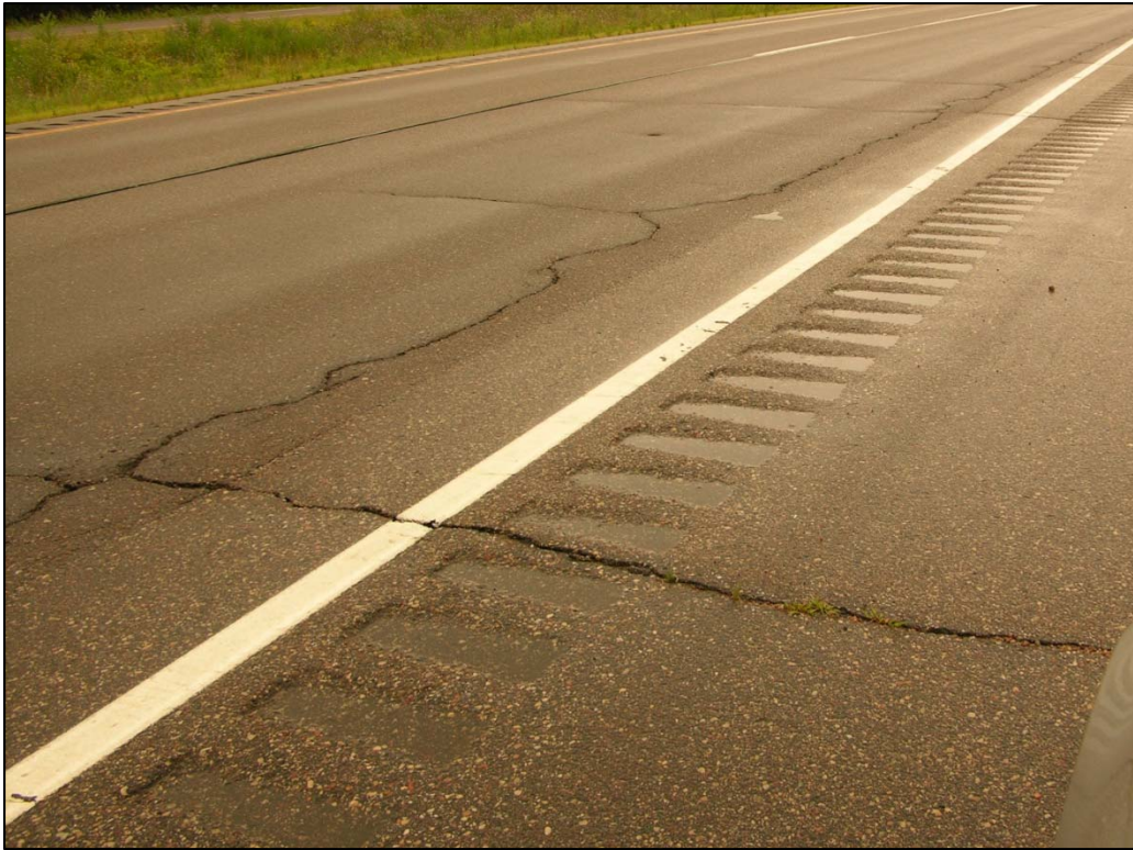
Figure 15. Control section cracking, July 2010.
