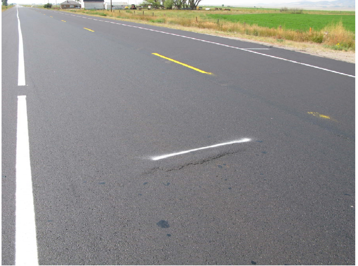
Figure 12. Bumps and Transverse Cracks at Station 150+00
