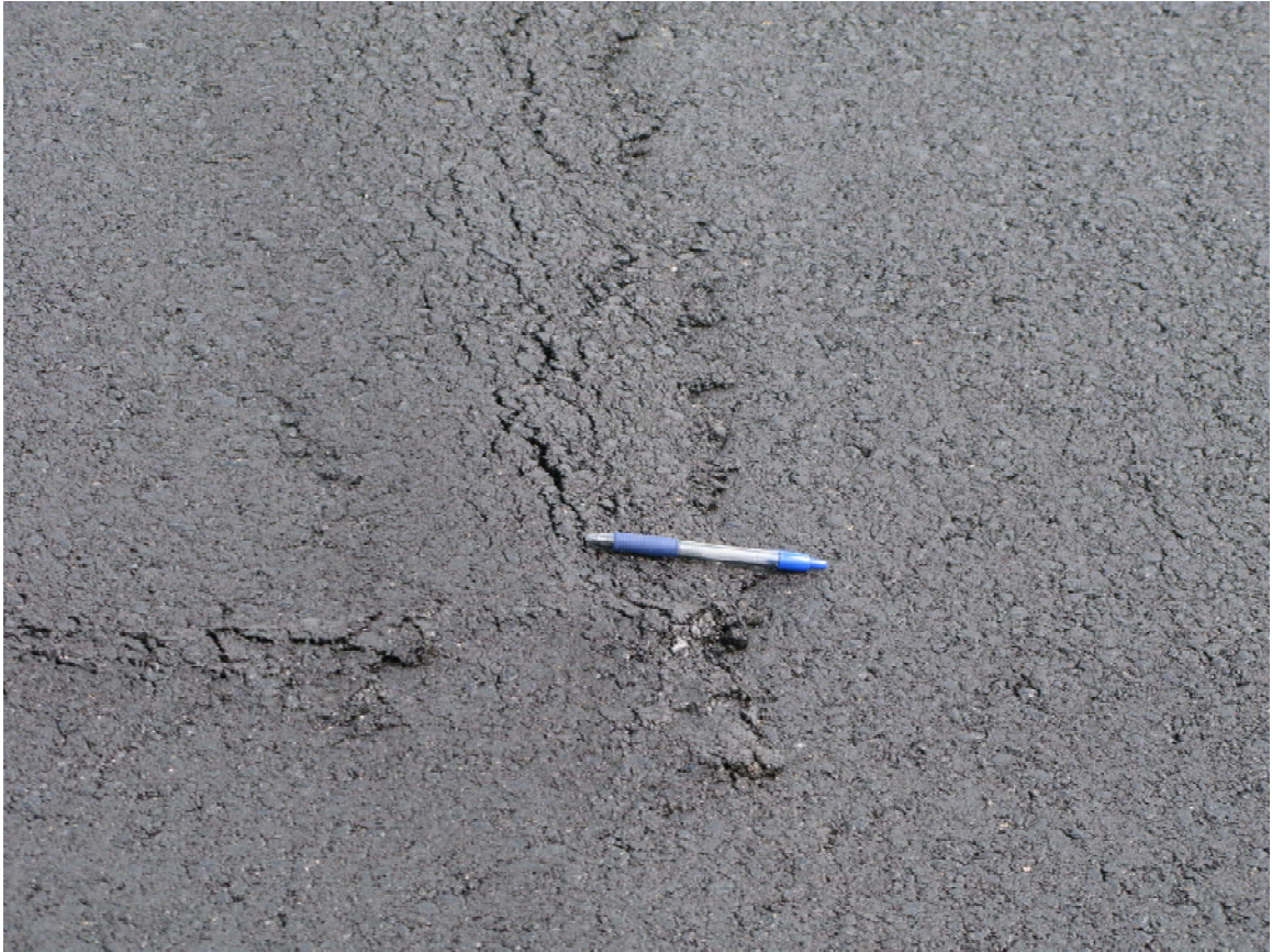
Figure 13. Bump and Transverse Cracks over Crack 271 on US 285
