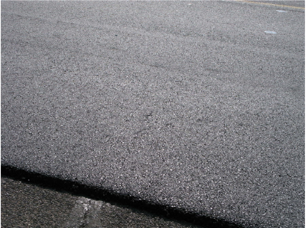
Figure 15. Transverse Crack Forming over Crack 201 Northbound US 285
