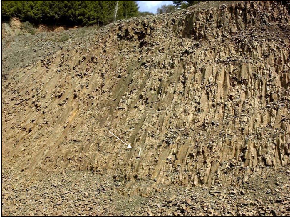
Close-up view of the jointing pattern, note the 4lb. maul for scale.
