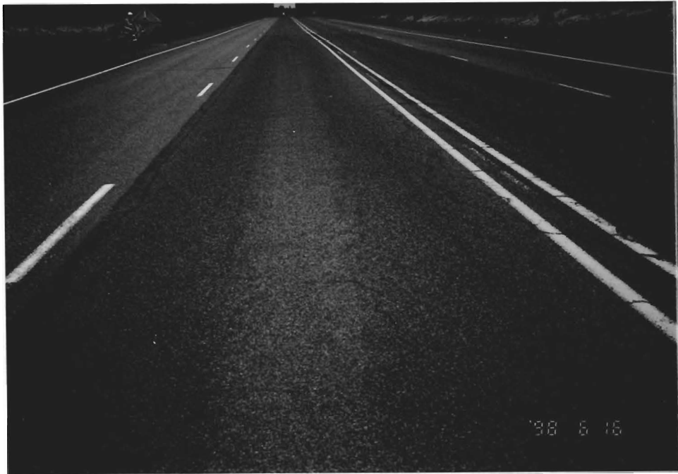
Figure 2.5: Wheeltrack Cracking on Plus Ride. About 7% of the wheeltracks were raveled. The newly constructed slow-moving-vehicle lanes are on the outside lanes. Location: MP 158.2
