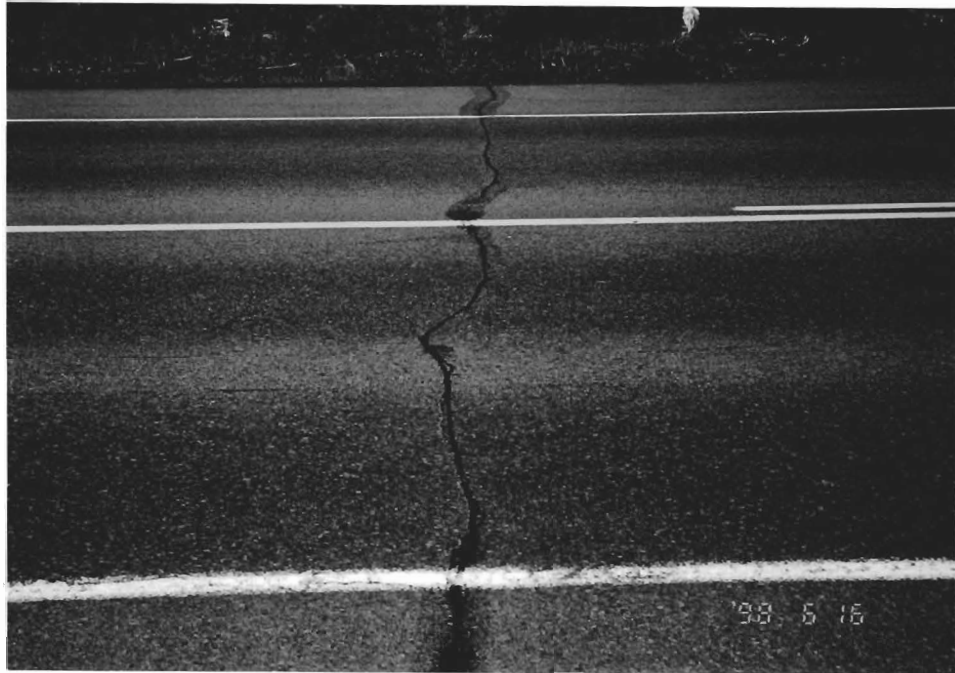
Figure 2.2a: Typical Transverse Crack that was Routed and Sealed. CA(P)-1 with Lime pavement is in the near lane, and CA(P)-1 pavement is in the far lane. Location: MP 161.5 looking west.
