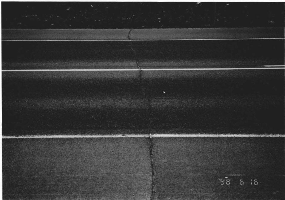
Figure 2.2.b: Typical Transverse Crack that was Routed, but Not Sealed. Arm-R-Shield is in the two travel lanes, and Class "C" with PaveBond and Lime is in the shoulder. Location: MP 158.6.
