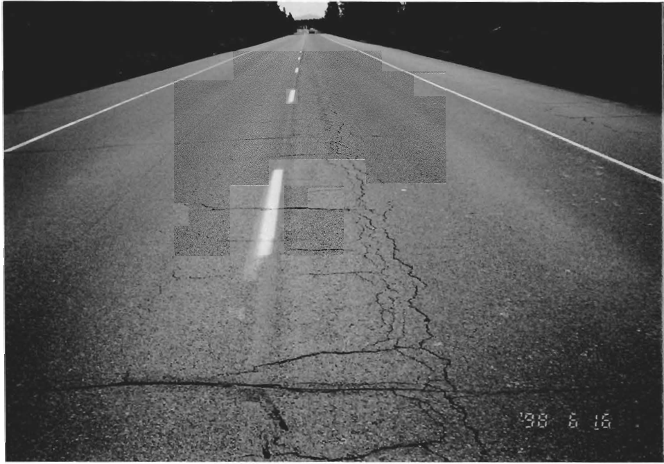
Figure 2.4: Typical Block Cracking and Fatigue Cracking. The Class "C" pavement is on the left, and the Class "C" with Lime and Pave Bond pavement is at the right. Location: MP 61.05 looking south.
