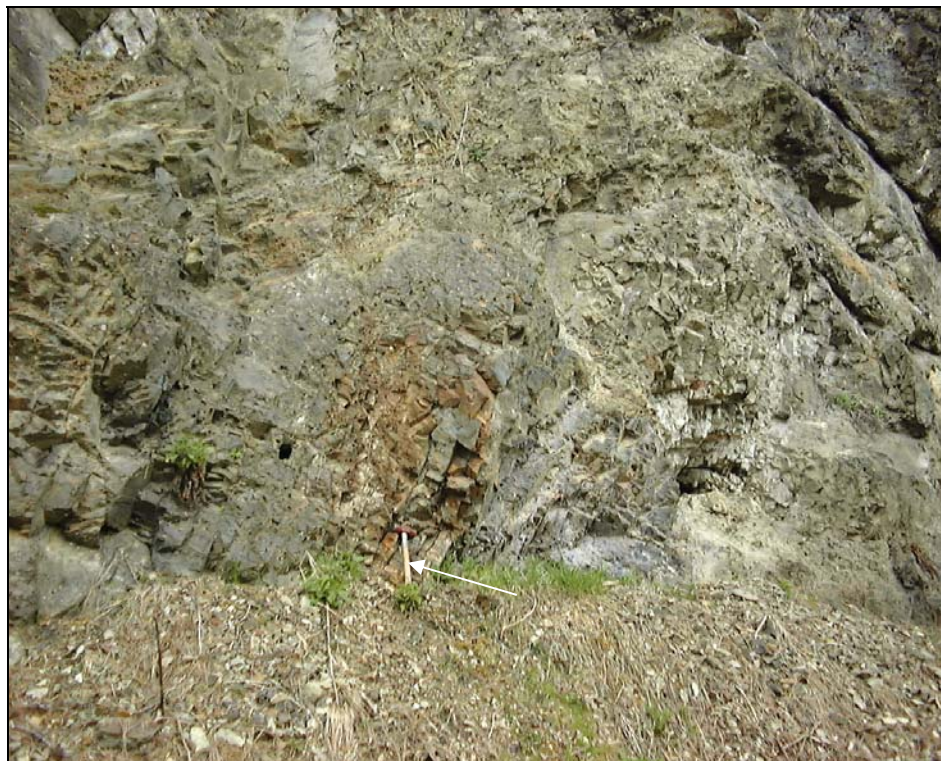
Close-up view of the fracture pattern along the face. Note the hammer for scale.
