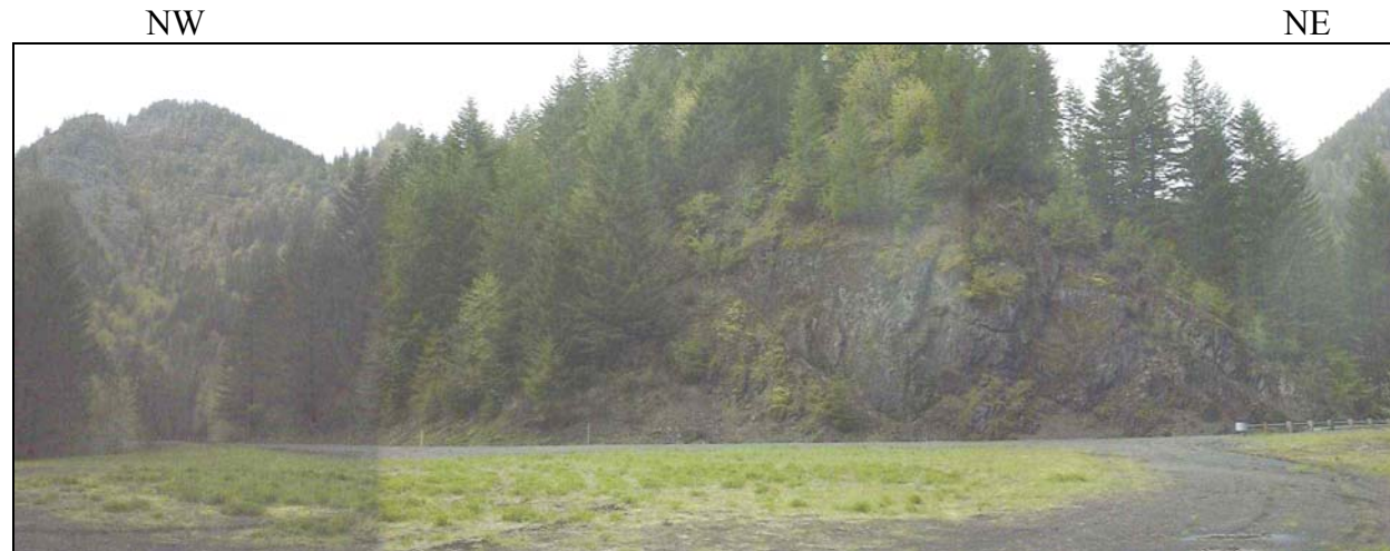
View to the north of the roadcut along Highway 6. The image was acquired from the stockpile site
