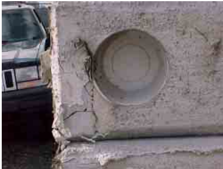
Figure 3.5: Cracks in a Block Removed in 1999.
