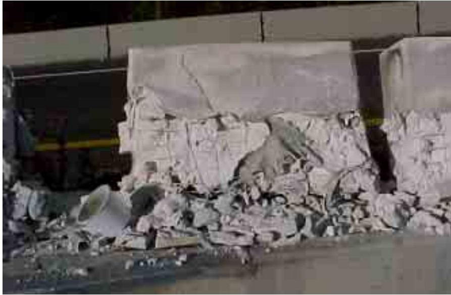
Figure 3.8: Blocks Crushed by Impact
