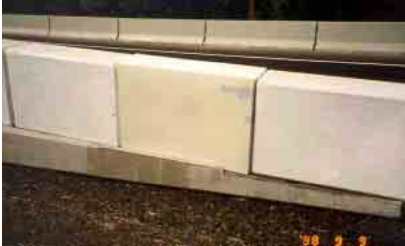
Figure 3.3: Waterproof Cover on Block
