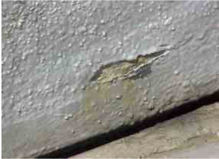
Figure 3.6: Tear in Garna-Thane Weatherproofing on Block
