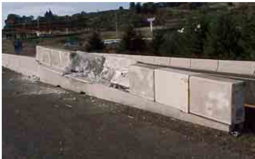
Figure 3.7: Damage from Vehicle Impact.
