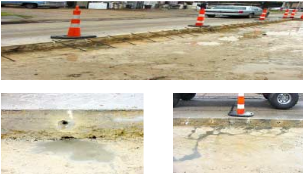
Figure 30 Pumping locations (Area 2)
