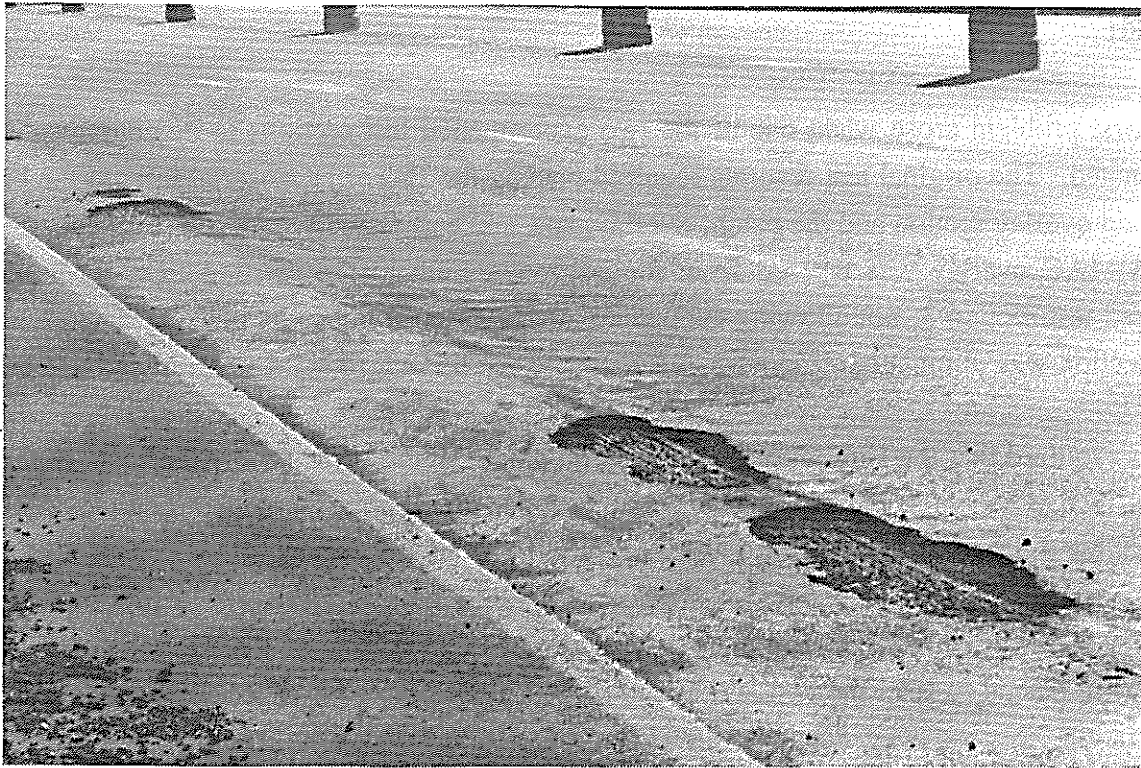
Figure 3. Extreme Raveling and spalling at HaTeLIT Interface.
