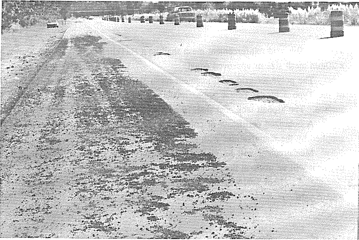
Figure 2. Extreme Raveling and spalling at HaTeLIT Interface.
