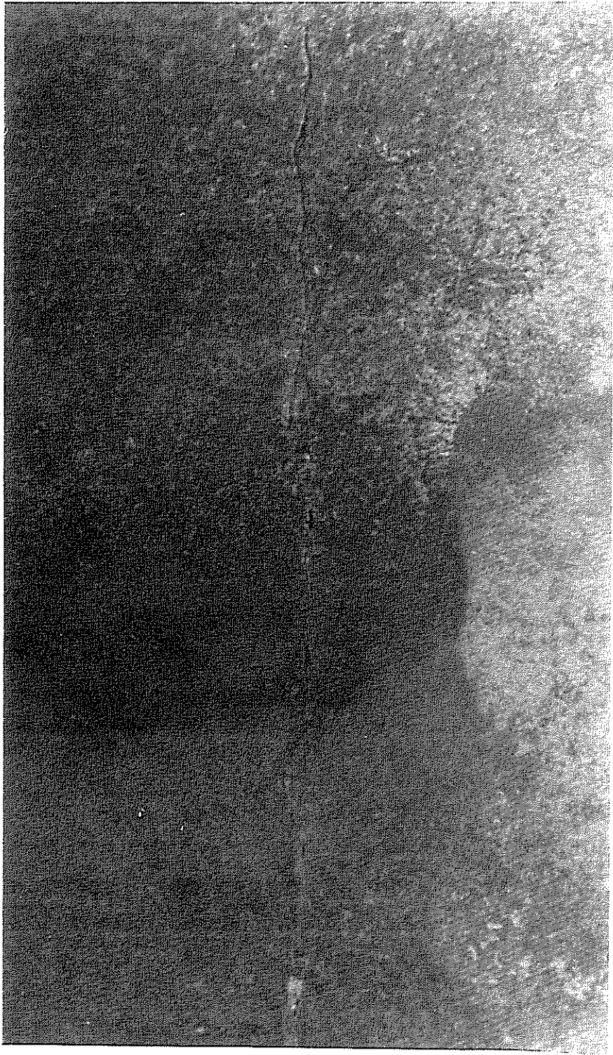
Figure 11 Typical hairline crack near waterline
