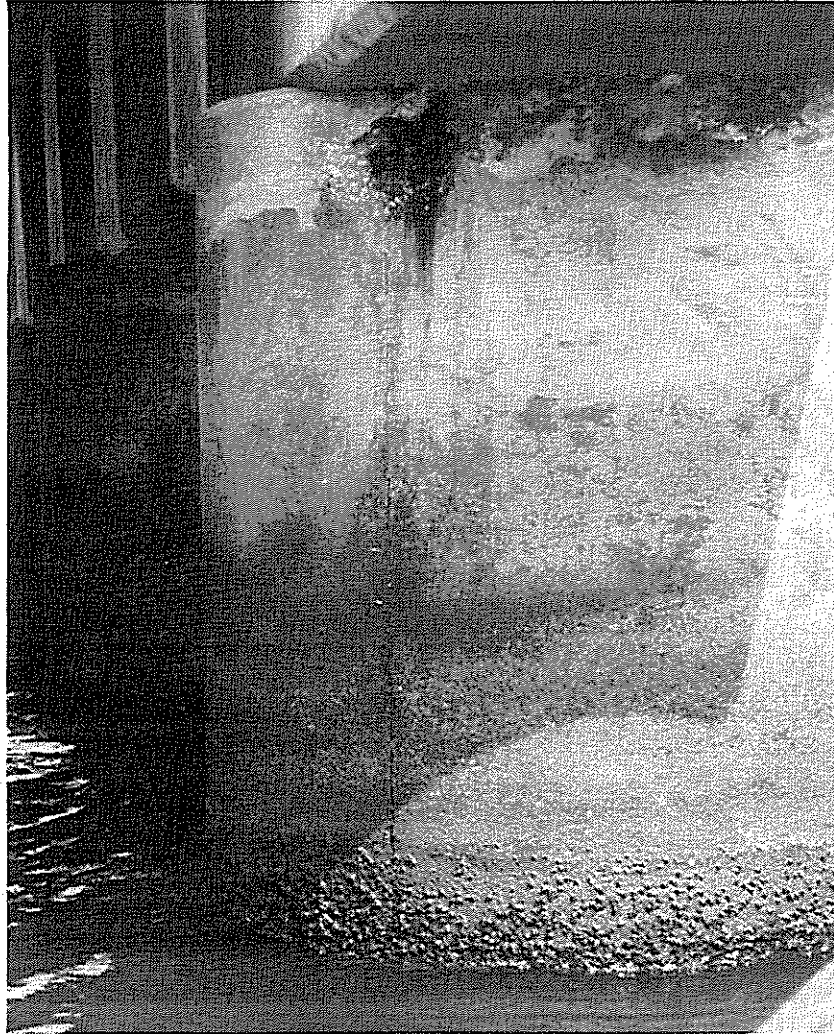
Figure 20 Seam in pile that looks like a crack
