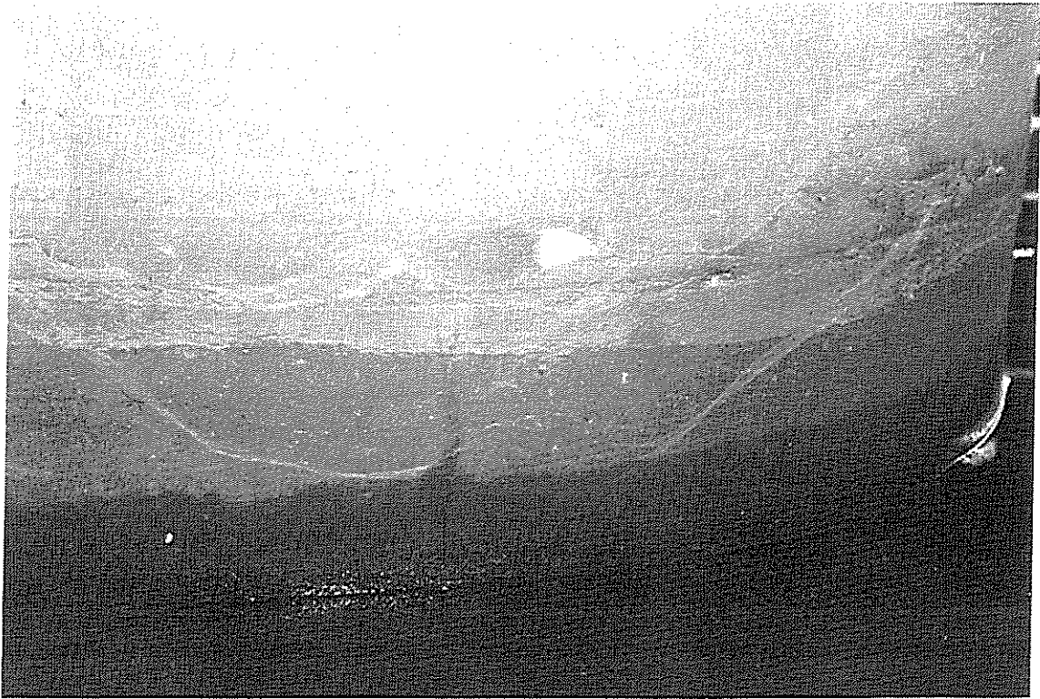
Figure 12 Typical hairline crack near waterline
