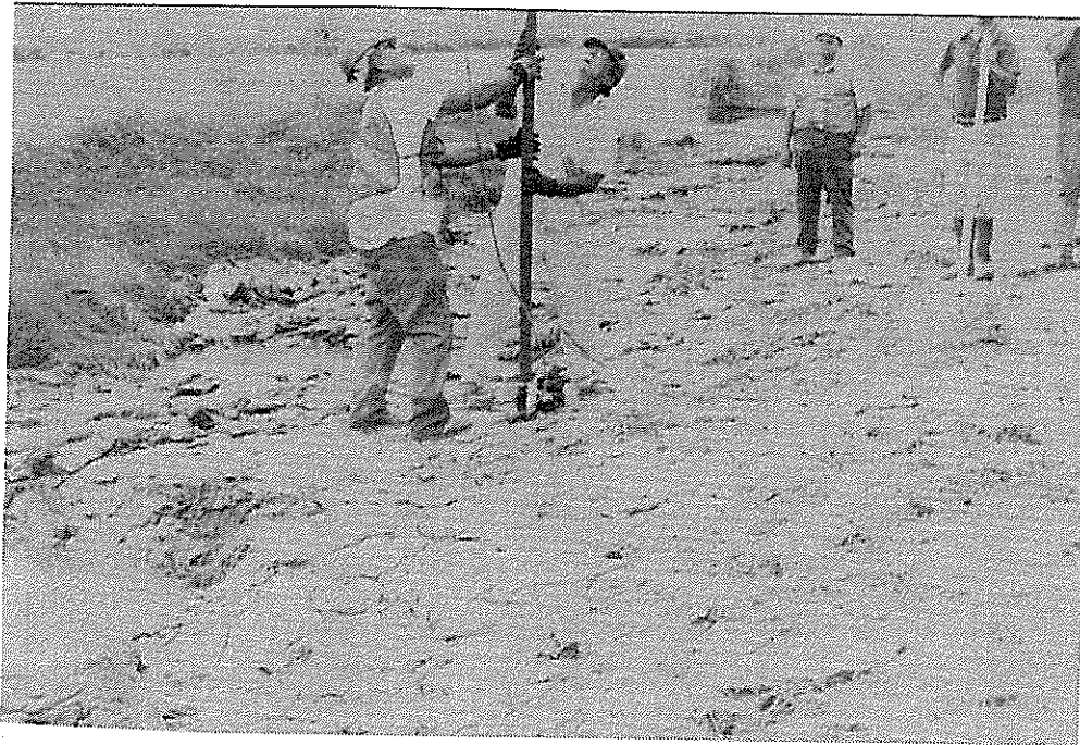
Figure 11. The external anodes were pushed into the ground using the Gradall shovel.
