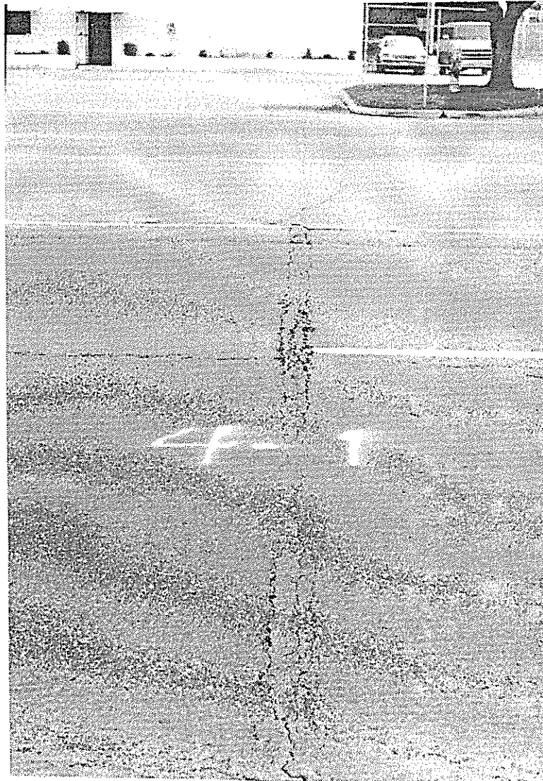
Test section 4. Conventional joint failure (with conventional asphalt cement).
