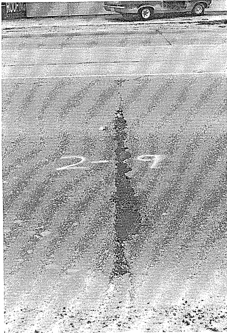
Test section 2. Taped-joint failure with maintenance patches (and conventional asphalt cement).
