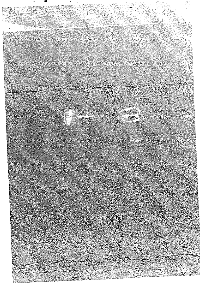
Test section 1. Less distressed taped-joint (with conventional asphalt cement).
