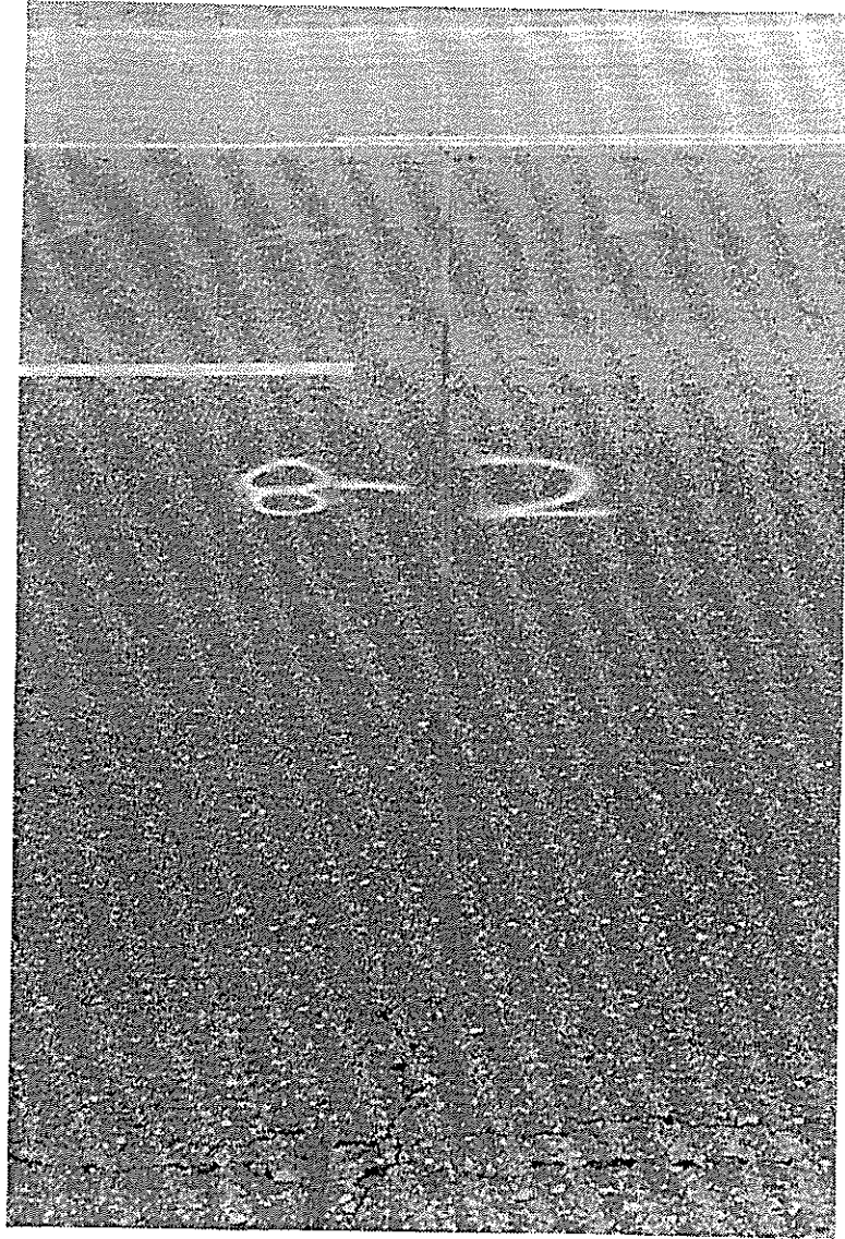
Test section 8. Distressed sawed and sealed joint (with conventional asphalt cement).
