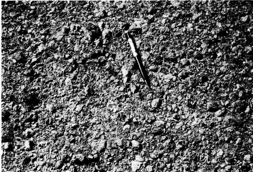
Figure 2 First Application Aggregate After Three Months of Service - no seal used.
