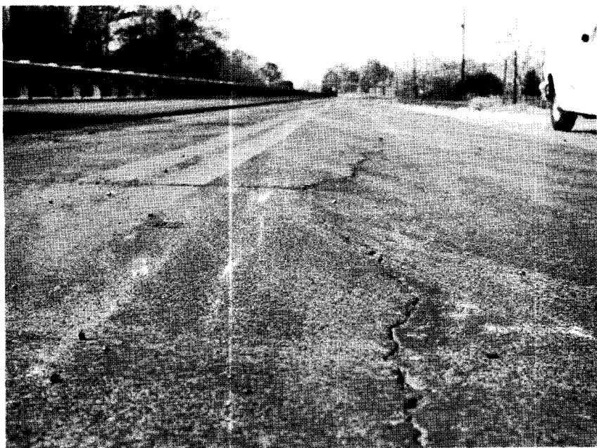
(A) Existing Pavement Crack before Overlay
