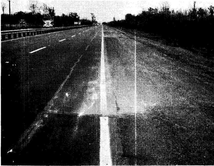
Figure 29 - Photograph of the Pumping and Cracking occurring on the Concrete Widening of the Eastbound Roadway 12 months after overlay
