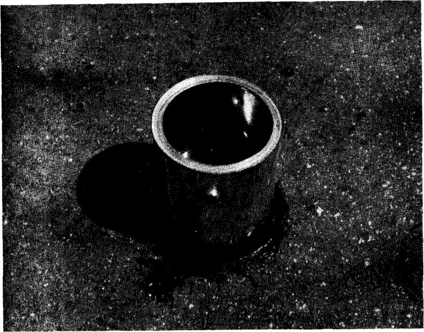
Photograph No. 7: Water Penetration Test on Reclamite Treated Section on La. 31 During September 1968
