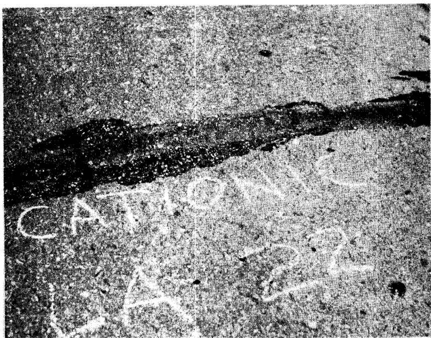
Photograph No. 3: RS-3K Treated Crack on La. 22 During September 1968
