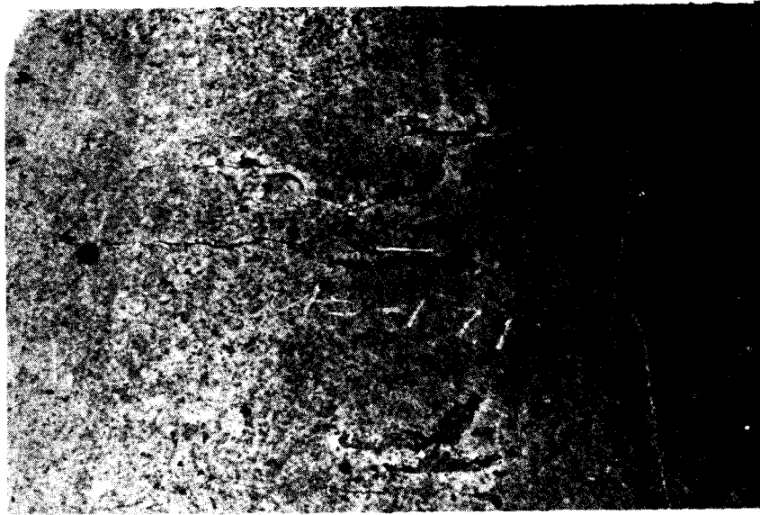
FIGURE 6 Bridge No. 1: Delamination has occurred to this area.
