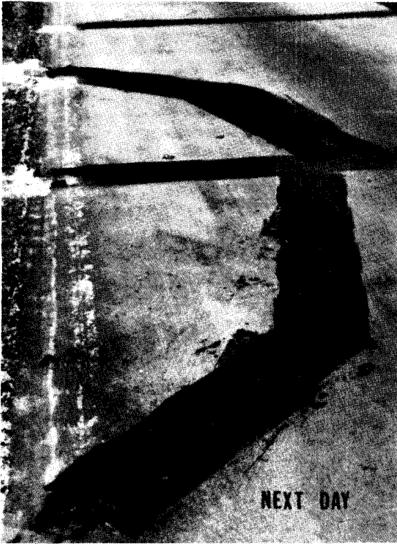
FIGURE 11 DISTRESSED CONCRETE PAVEMENT IN TEST SECTION - U. S. 61
