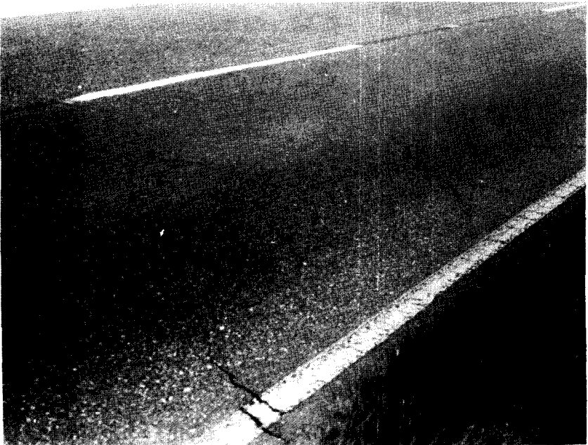
FIGURE 12 REFLECTION OF ORIGINAL CRACK SHOWN ABOVE
