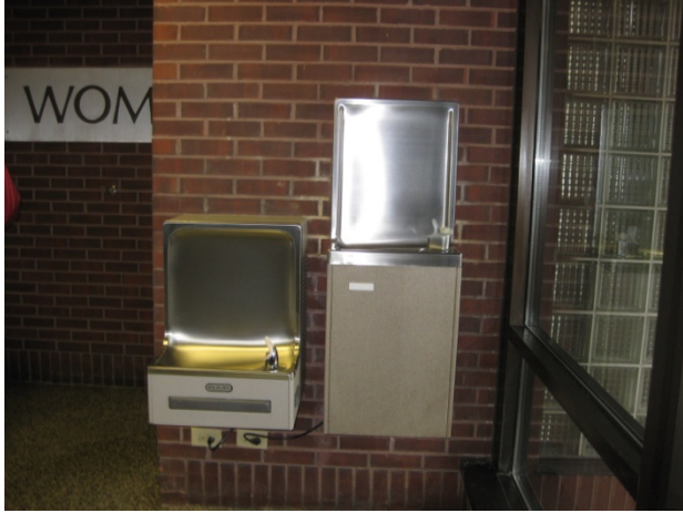
Figure 35. Water cooler of Pride of the Prairie rest area.
