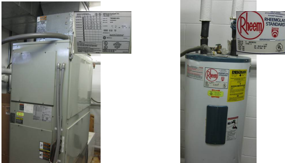
Figure 32. Air conditioning and water heater units of Pride of the Prairie rest area.
