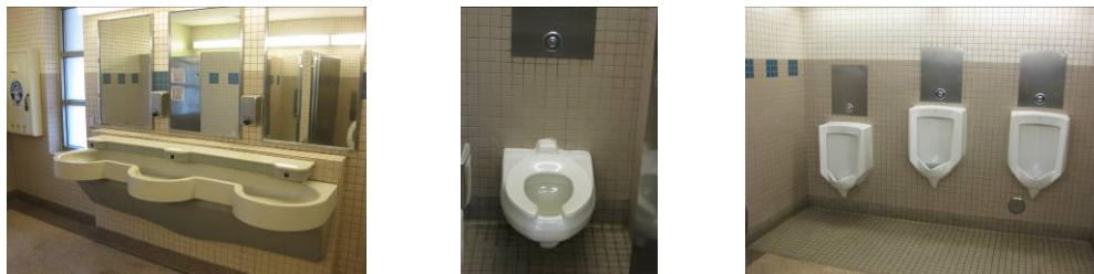
Figure 31. Water fixtures of Funks Grove rest area.
