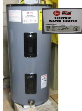
Men's bathroom water heater
