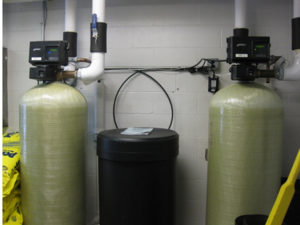
Figure 33. Water treatment pressure filters of Pride of the Prairie rest area.
