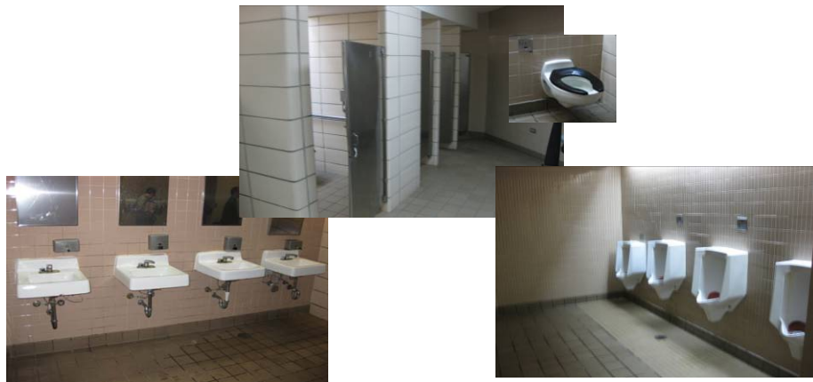
Figure 26. Water fixtures of Prairie View rest area.
