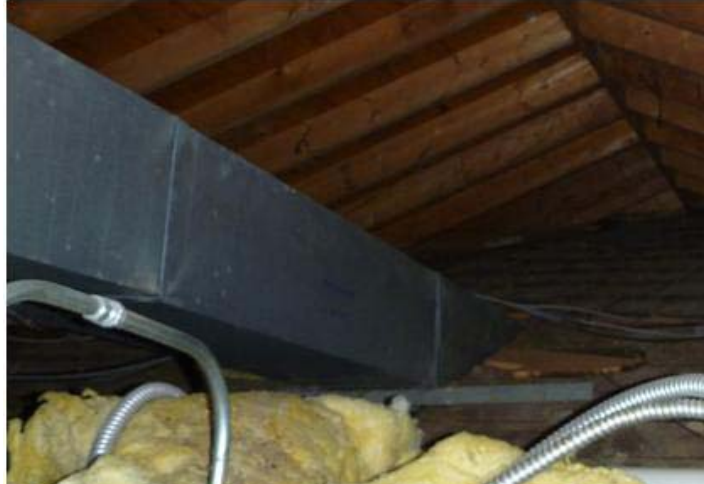
Figure 3: Uninsulated Duct Showing Signs of Air Leakage in the Vented Attic Space
