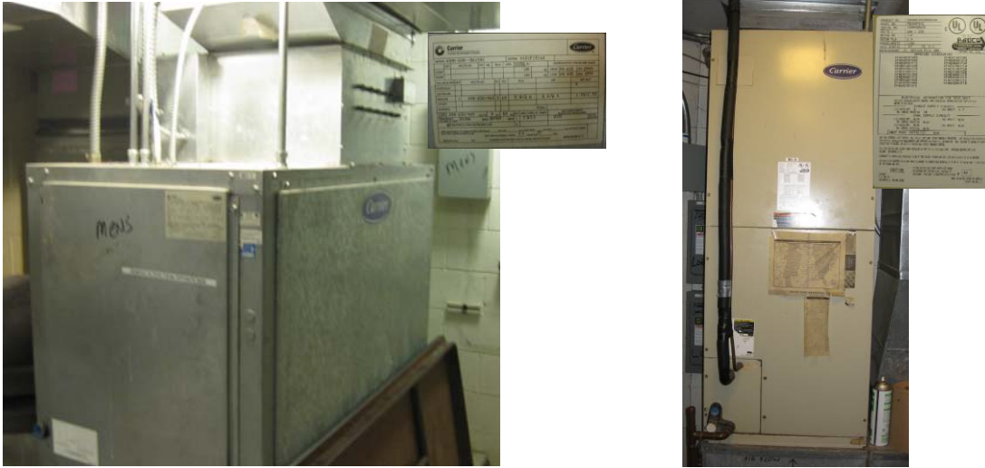
Figure 28. Two models of the air conditioning units in Funks Grove rest area.
