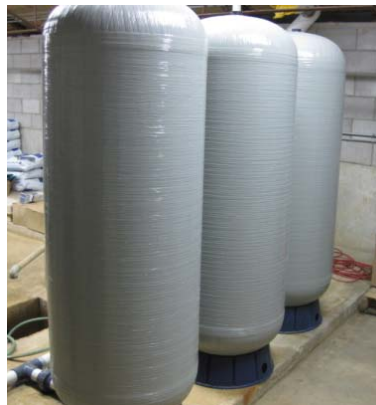
Figure 25. Three pressure filters of the water treatment system of Prairie View rest area.
