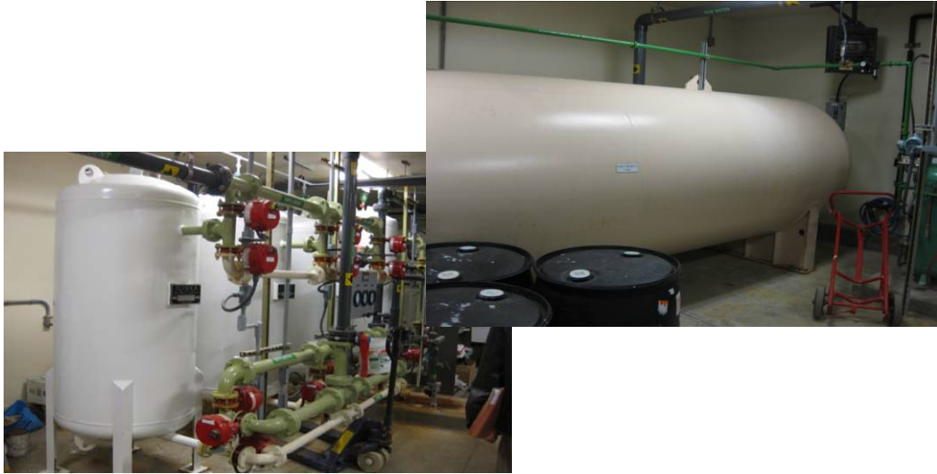
Figure 29. Pressure filters and hydropneumatic tank of Funks Grove rest area.
