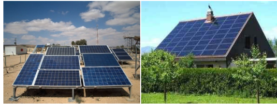
Figure 44. Solar panels of photovoltaic systems.
