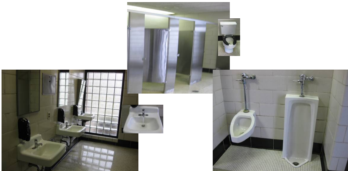
Figure 36. Water fixtures of Pride of the Prairie rest area.
