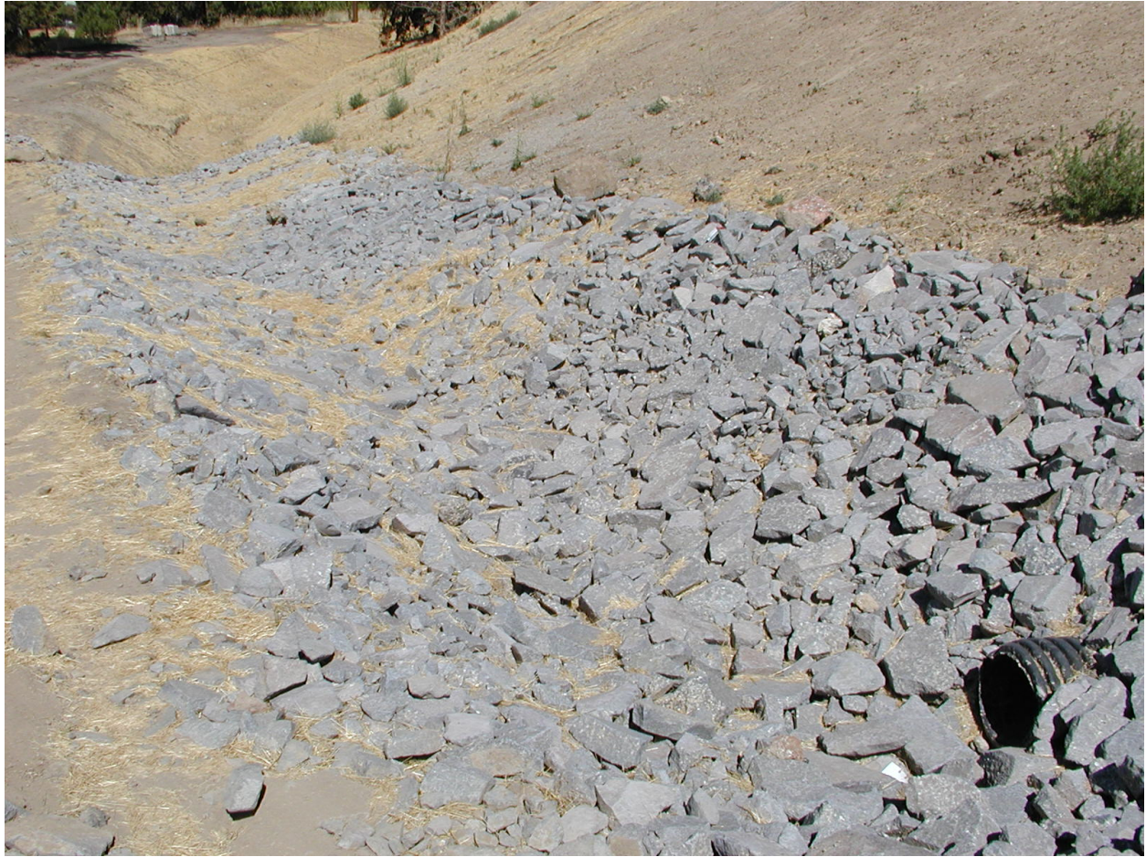
Rock lined ditch to carry water from middle section of Highway 20 in Bend, Oregon beside Pilot Butte to detention ponds and dry wells.
