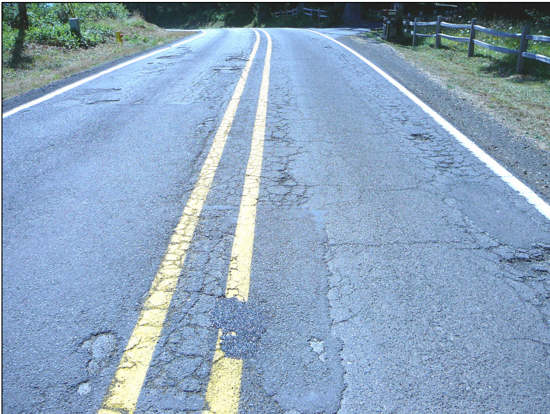
Figure 4.9: Poor roadway conditions
