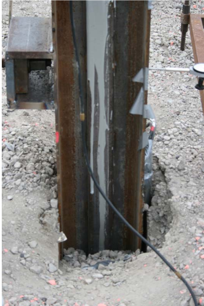
Figure 36: Gap at 445-kN (100,000-lb)
