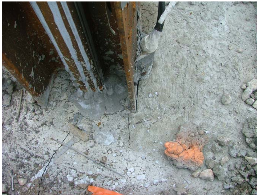
Figure 48: Cracking at 556 kN-667 kN (125,000 lb-150,000 lb)
