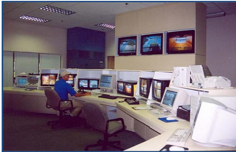
Figure 3. CGT Control Room Circa 1997
