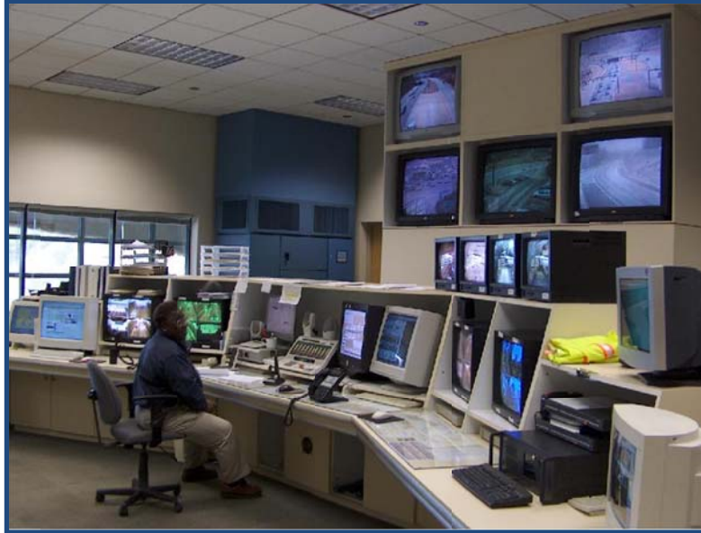
Figure 4. CGT Control Room Circa 2003
