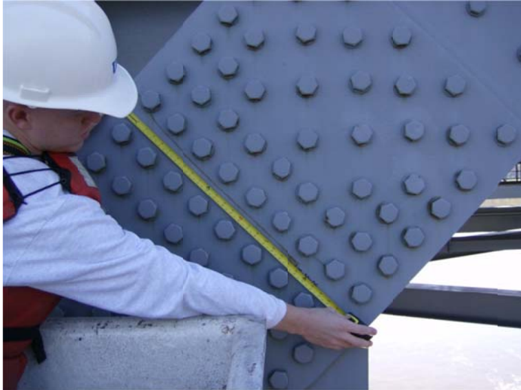
Figure 4. Crack in 3/8-Inch Thick Splice Plate at Panel Point L12' on the Downstream Truss of the Westbound Bridge (Courtesy of URS Corp).
