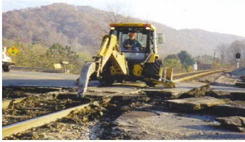
KY 3 Condition prior to rebuild
