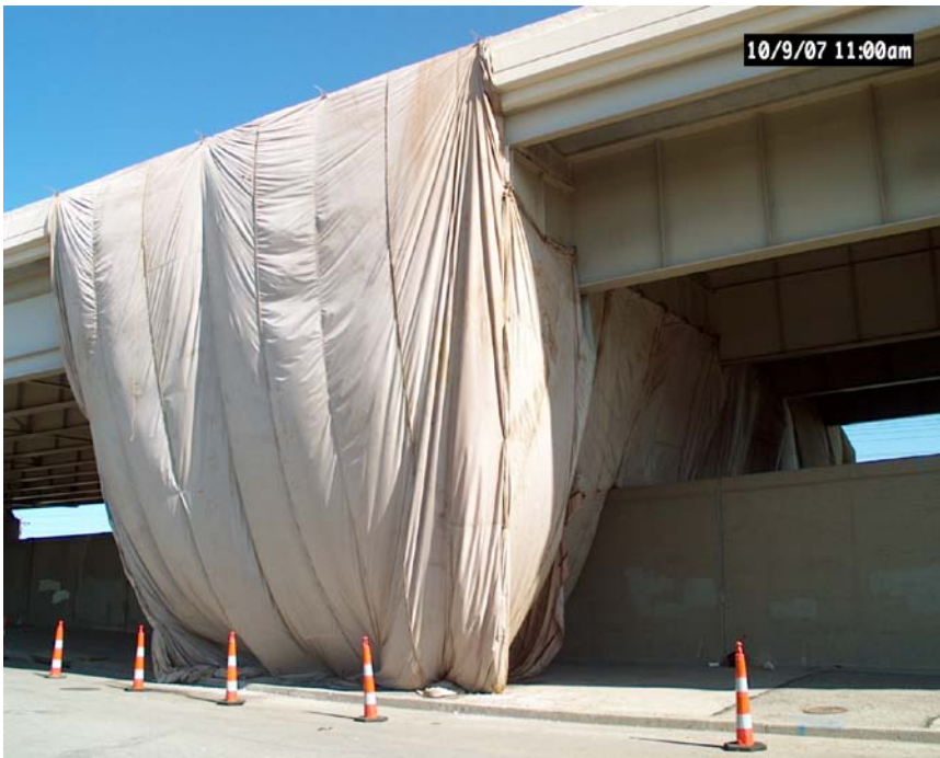
Figure 8. Grounded containment enclosure splitting a retaining wall at bridge B00282 on I-64 between 22 nd Street & Northern Parkway (Eagle Painting).
