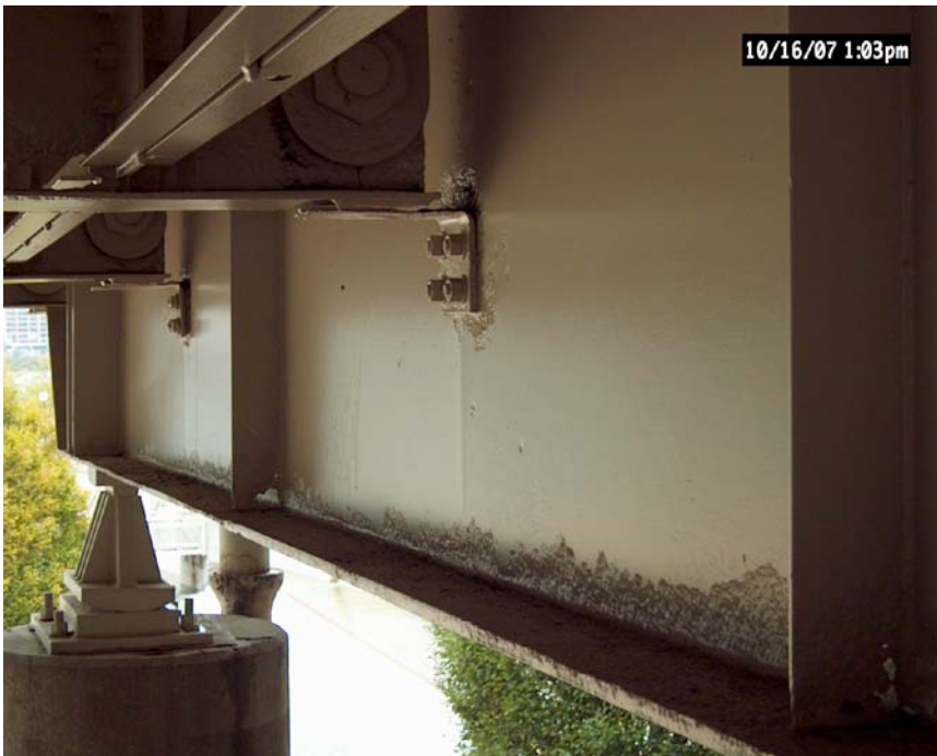
Figure 20. Corrosion damage to a floor beam highlighted by application of the new coating.
