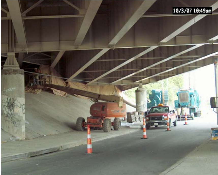
Figure 9. Containment enclosure being installed at I-64 bridge abutment on B00285 (Bridges 'R Us).
