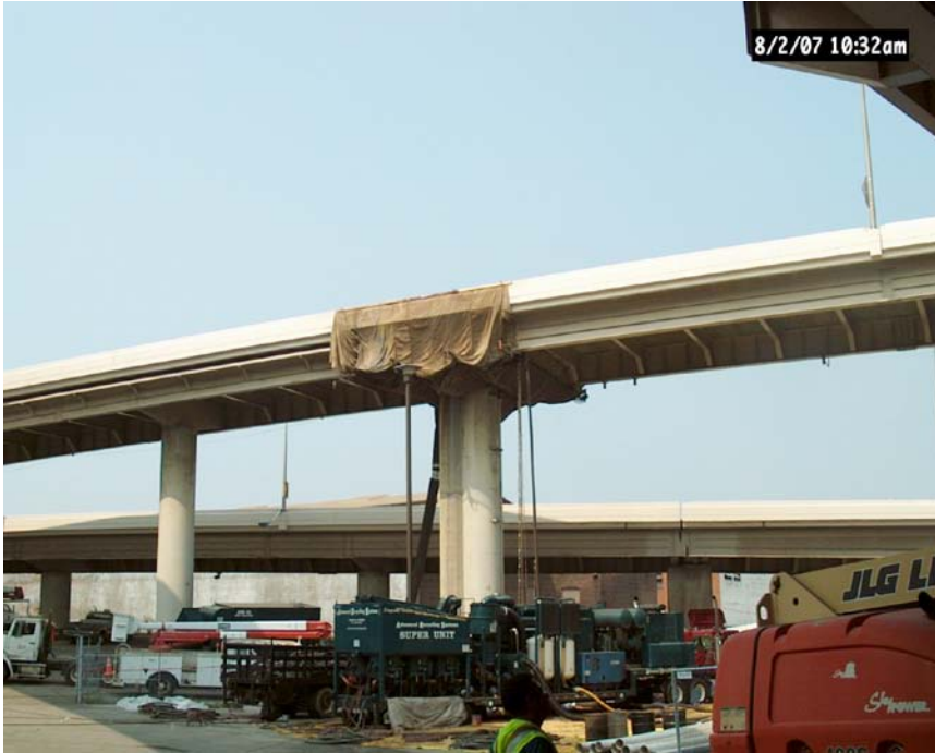
Figure 7. Elevated containment enclosure at bridge B00299 the 9 th Street Interchange to I-64 eastbound (Bridges 'R Us).
