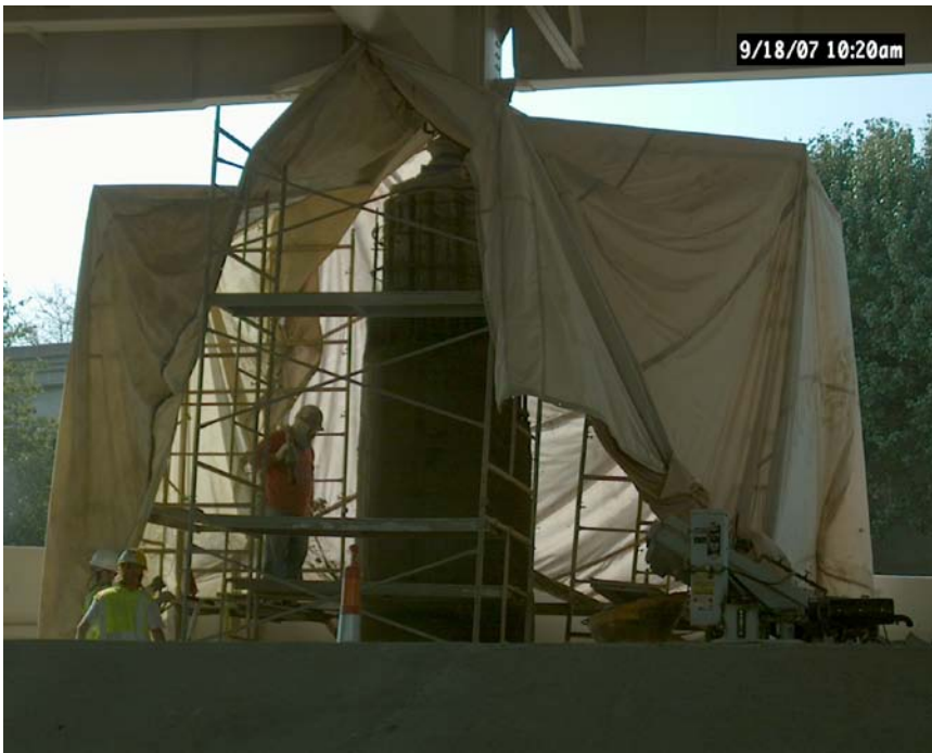
Figure 4. Crew installing containment enclosure at a joint area prior to cleaning and painting operations.
