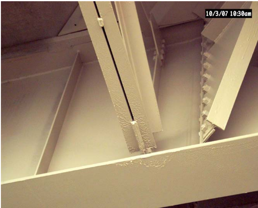
Figure 18. Areas on the bottom of cross bracing and a flange that have excessive paint build-up.
