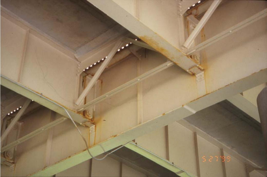
Figure 1. Corrosion on underlying structural steel under open deck joint (1999).
