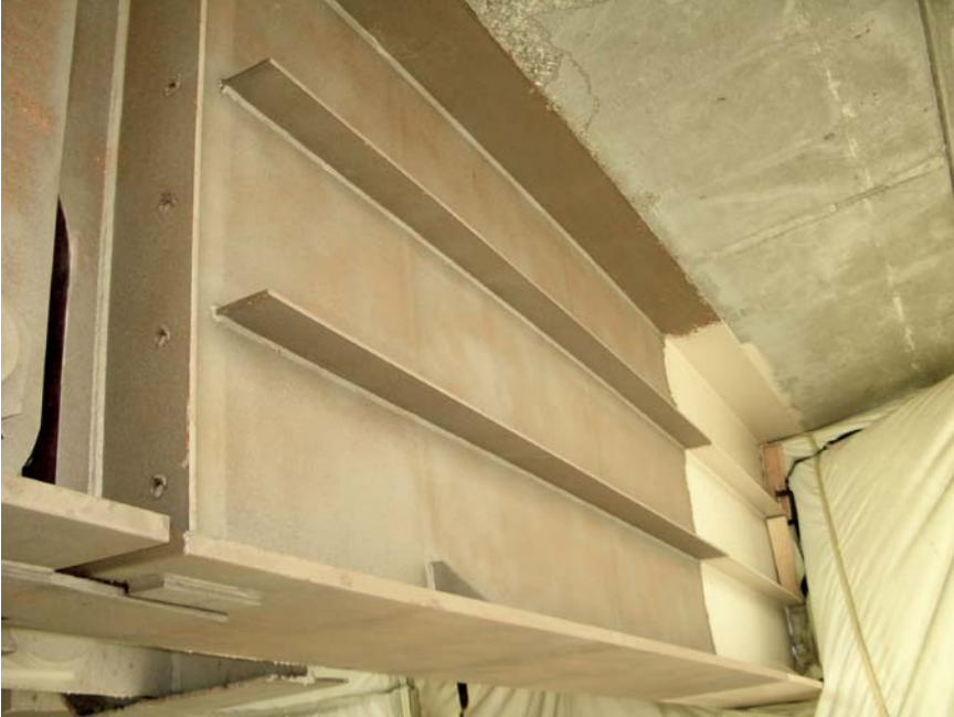
Figure 15. Area near joint that has been blasted and partially painted near a bulkhead.
