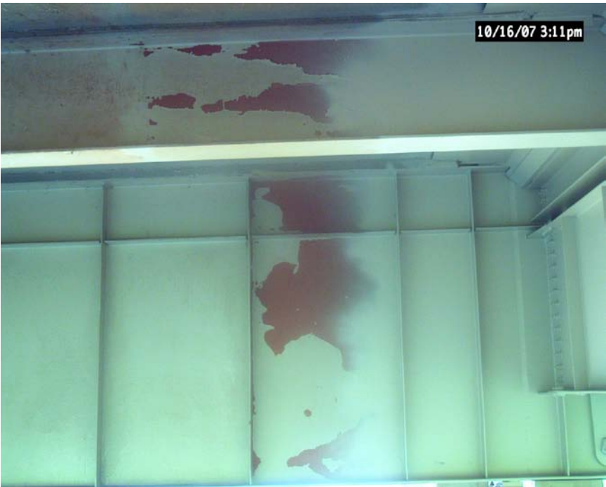
Figure 16. Area near cross-frame repair that has been power tool cleaned and partially painted on bridge B00292.
