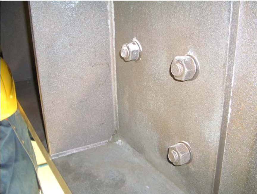
Figure 14. Improperly blast-cleaned bolts with excessive rust residue that had to be re-blasted prior to painting.
