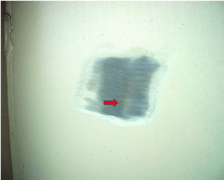
Figure 36. Rust formation in pit at steel substrate (April 2009).
