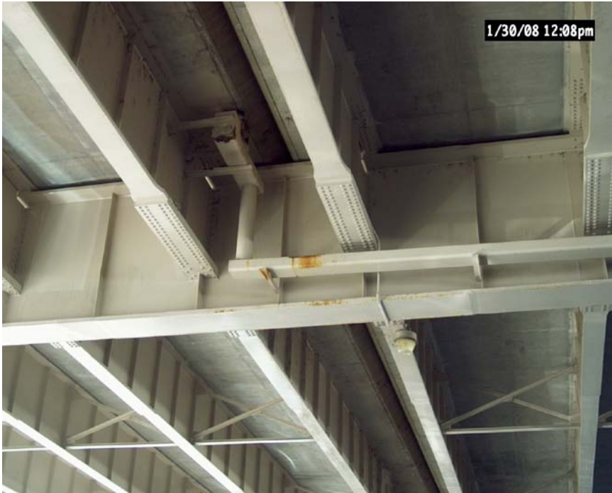
Figure 29. Rust-back and staining due to leakage from longitudinal deck joint (January 2008).
