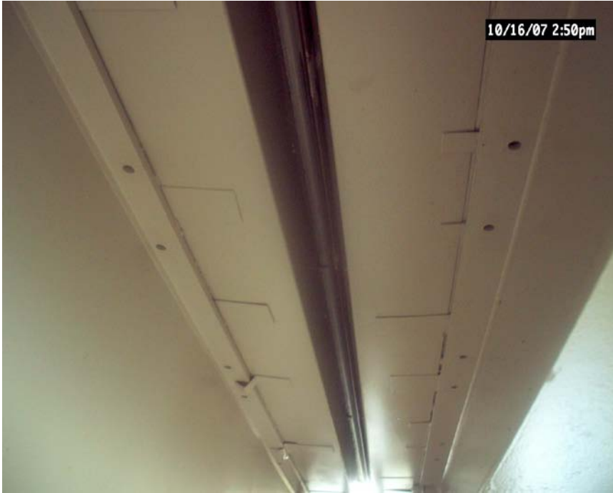
Figure 17. Coating on added steel under decks that is part of the new closed deck joints.
