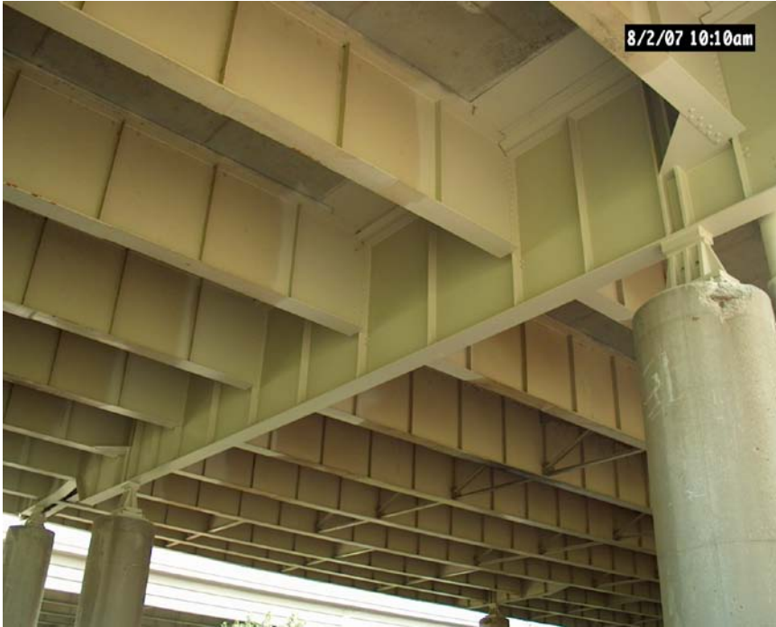
Figure 23. An area approximately five feet from joint that was cleaned and painted by Eagle Painting. Note the color difference between the existing and new paint.
