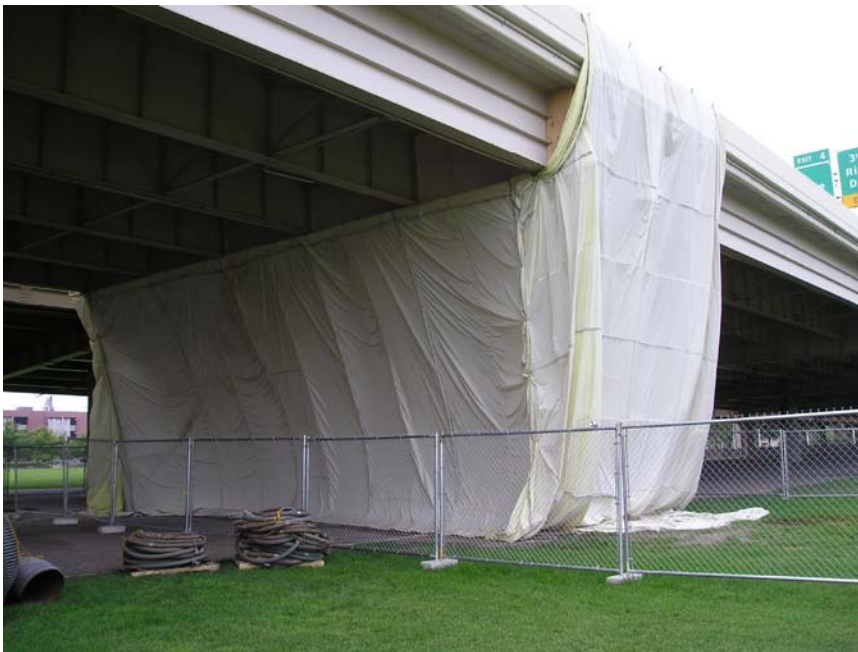
Figure 6. Typical containment by Eagle Painting during blasting operations at the Riverfront Park. Note the concave shape of the containment walls (negative pressure).
