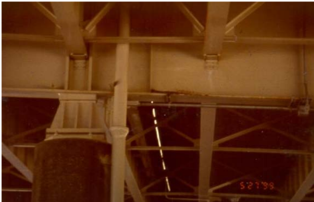
Figure 2. Debris build-up on lower flange due to presence of open deck joint (1999).
