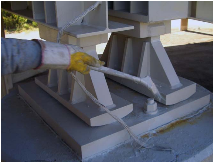
Figure 22. Worker using a brush to touch-up the coating on a bearing rocker.
