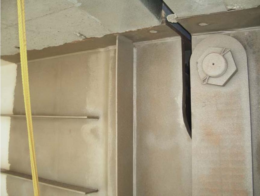
Figure 13. Blast-cleaned area at expansion joint ready for painting. Note the blast finish on the hanger and beam ends has visible traces of lead paint and mill scale.
