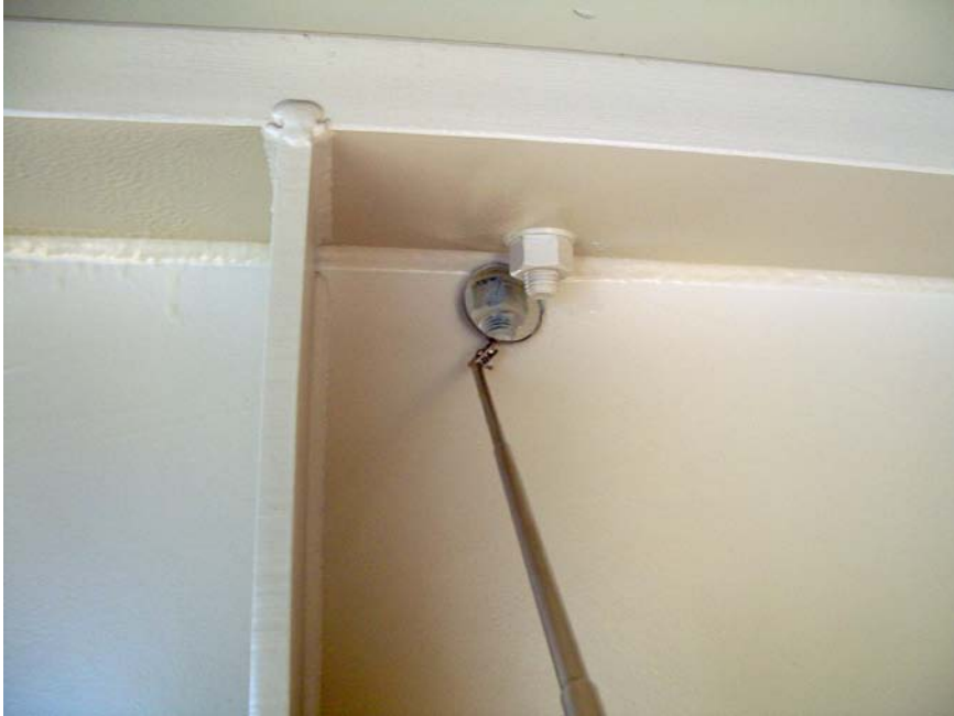
Figure 19. A missed spot on the backside of a fastener detected after painting.
