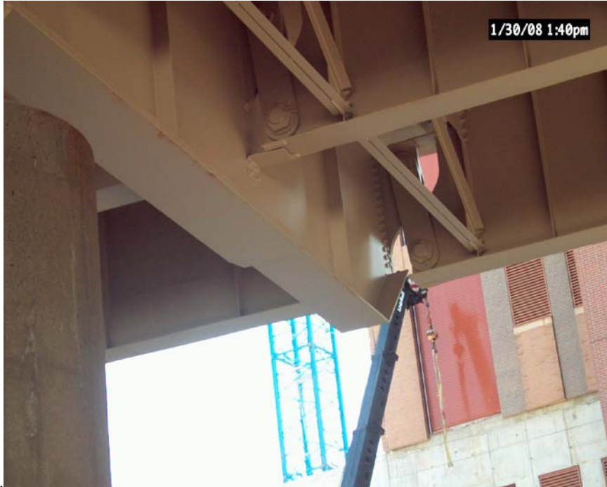
Figure 27. Rust-back at edge of a lower flange on a floor beam at an expansion joint (January 2008).
