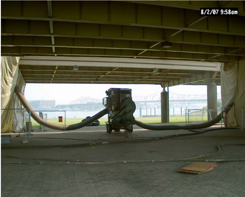
Figure 5. Vacuum system for applying negative pressure to containment enclosure and for collecting airborne fines. Unit is connected to two enclosures by large ducts.
