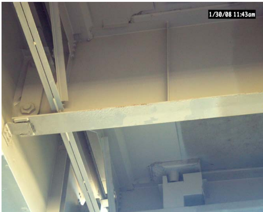
Figure 28. Zone painted area showing rust-back on edge of lower flange of a girder (January 2008).
