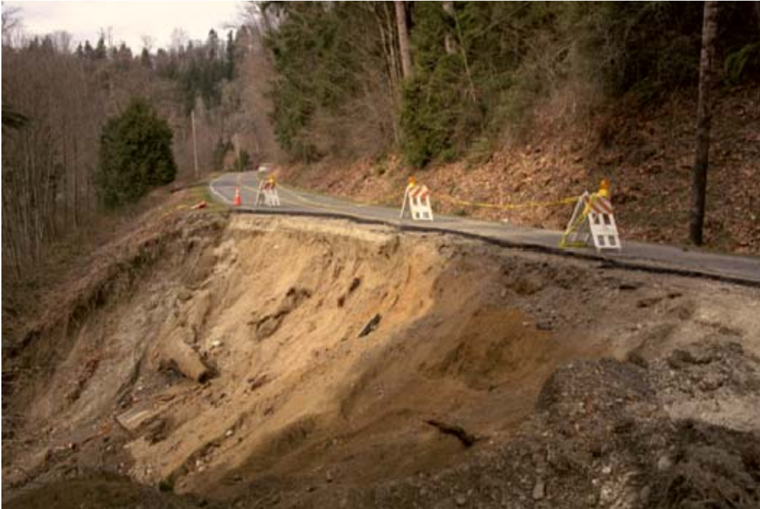
Figure 1-8. Road damage caused by slope failure during the 2001 Nisqually, Wash., earthquake.
