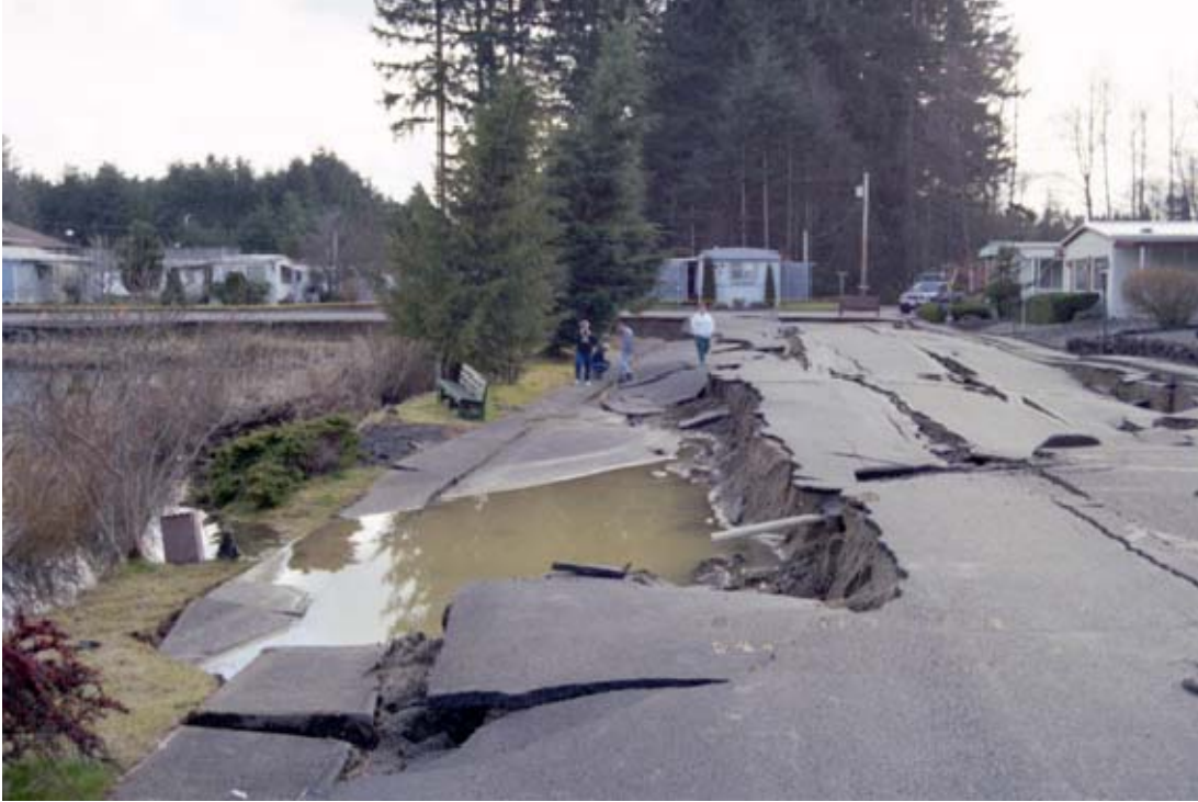
Figure 1-7. Road damage caused by liquefaction during the 2001 Nisqually, Wash., earthquake.
