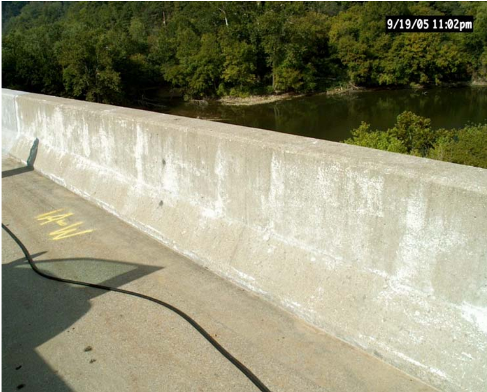
Figure 13. Barrier wall panel on US 676 connector over KY river in Frankfort, KY prior to surface preparation and coating
