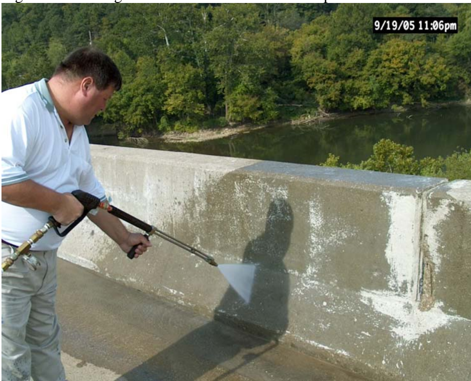
Figure 16. Pressure washing the barrier wall with a 15° fan tip at around 2500 psi
