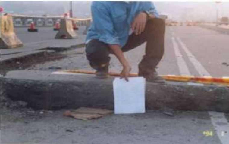
Figure 21 Moderate Damage. Approach settlement at the abutment. (2)
