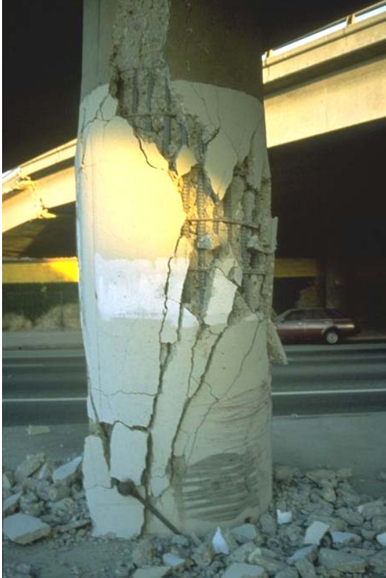
Figure 66 Severe Damage. Shear failure in column. (1)
