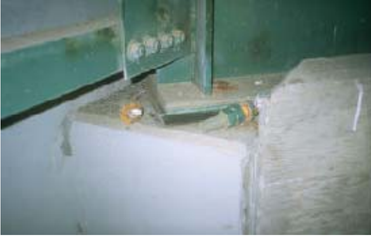
Figure 56 Moderate Damage. Sheared anchor bolts. (1)
