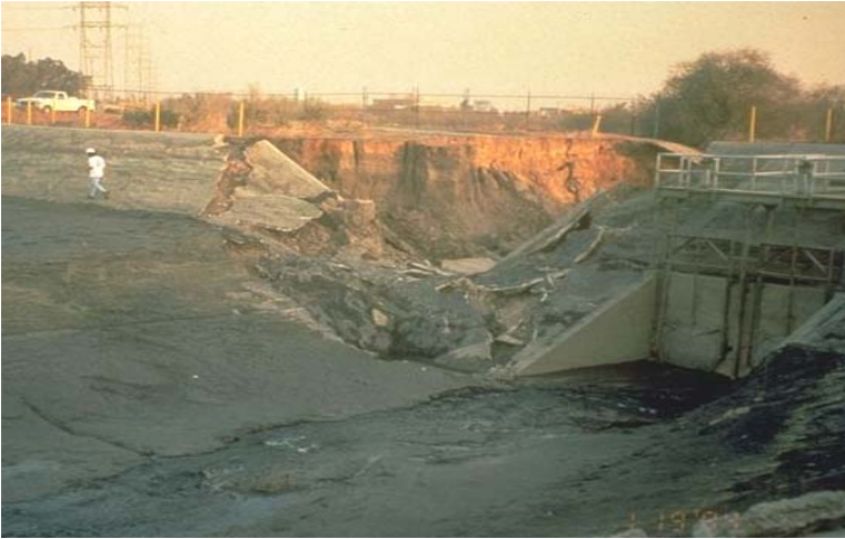
Figure 23 Total Failure. Embankment settlement. (1)
