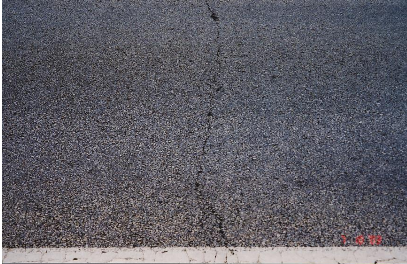
Figure 6a. Transverse Cracking (Slight).
