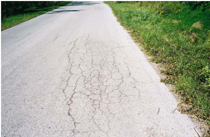
Figure 2b. Alligator Cracking (Moderate)
