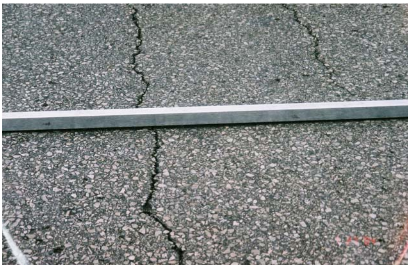
Figure 6c. Transverse Cracking (Severe).
