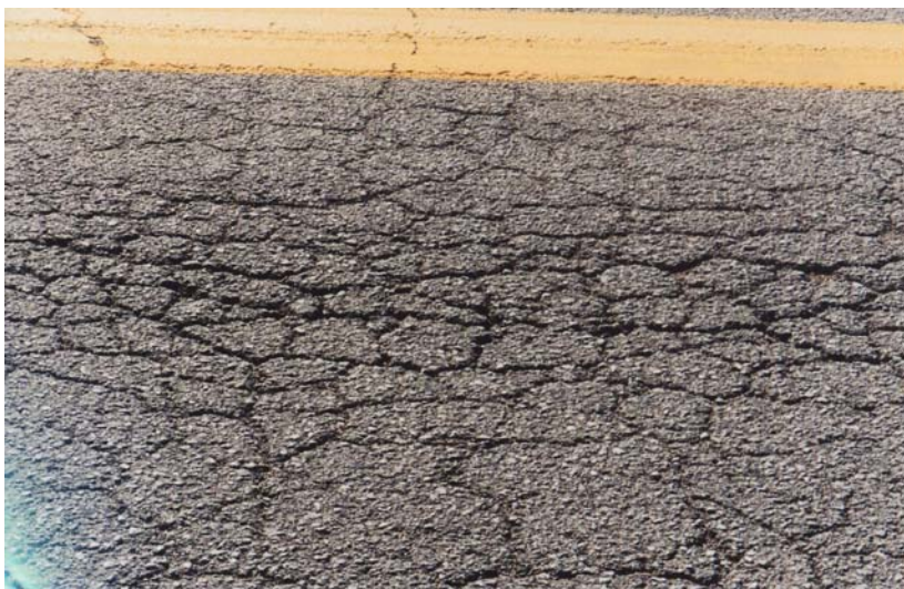
Figure 2c. Alligator Cracking (Severe)
