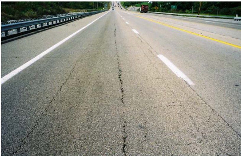
Figure 1c. Longitudinal Cracking (Severe)
