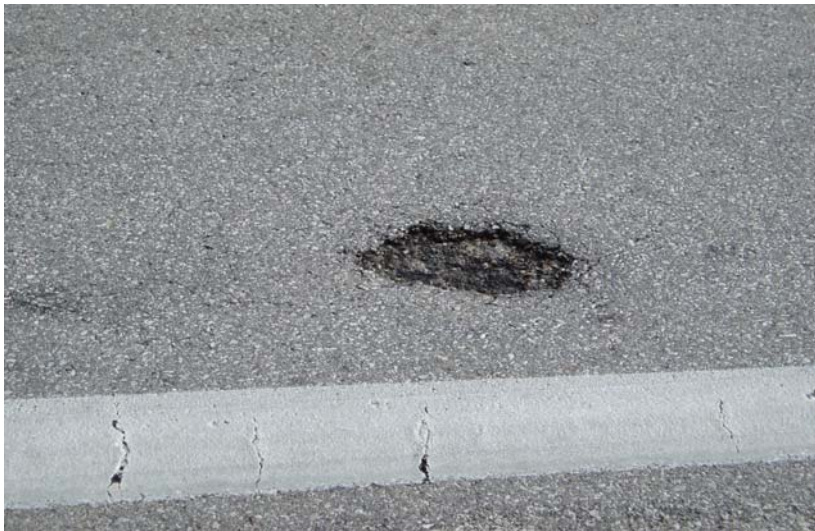
Figure 10a. Pothole (Slight)
