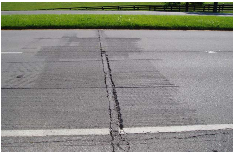
Figure 5c. Reflective Cracking (Severe).
