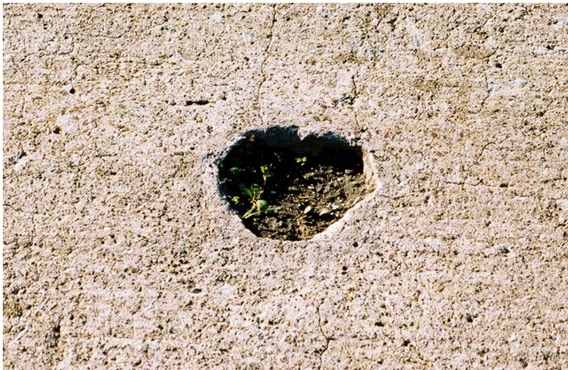
Figure 17c. Pop Out (Severe)
