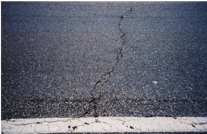
Figure 6b. Transverse Cracking (Moderate).
