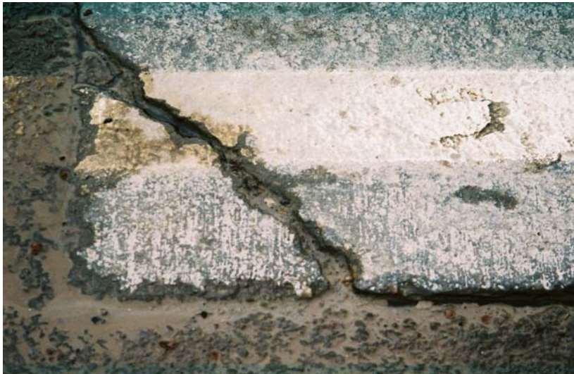
Figure 11b. Corner Cracking (Moderate)
