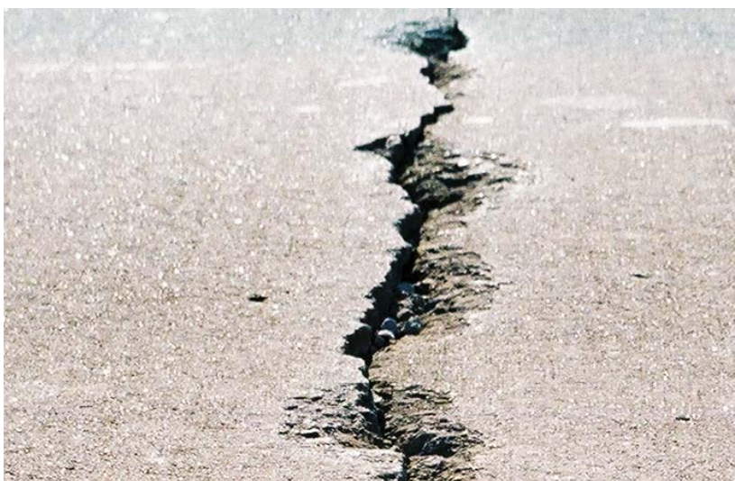
Figure 12c. Transverse Crack (Severe)
