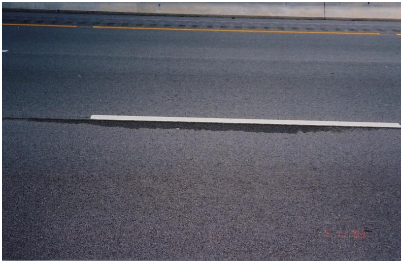
Figure 9a. Water Pumping (Slight)
