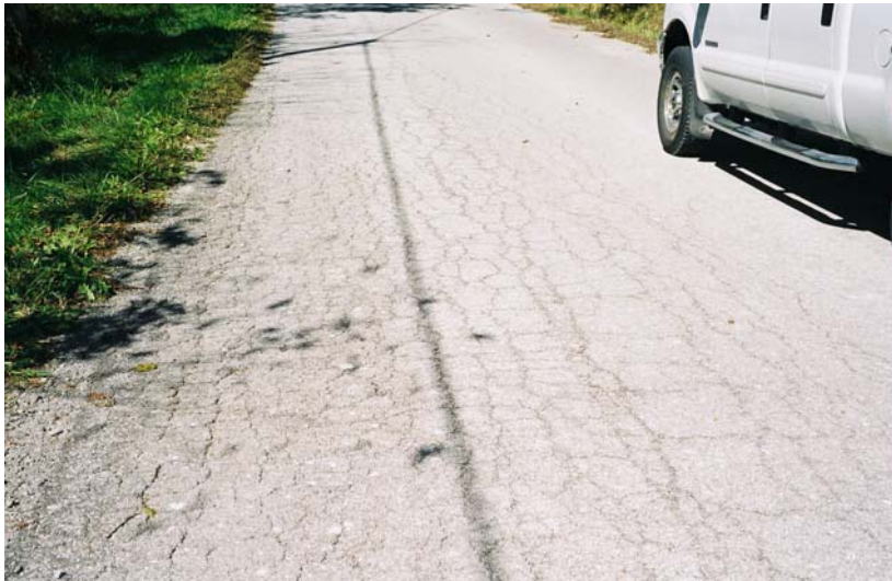
Figure 2a. Alligator Cracking (Slight)
