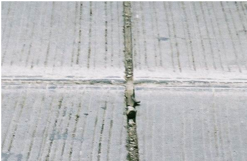
Figure 18b. Joint Seal Failure (Moderate)
