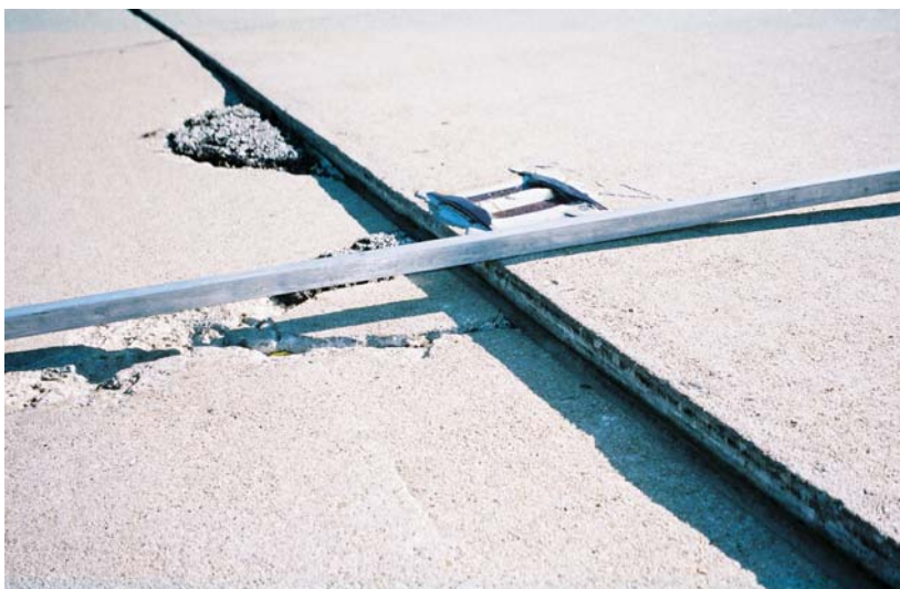
Figure 16c. Transverse Faulting (Severe)
