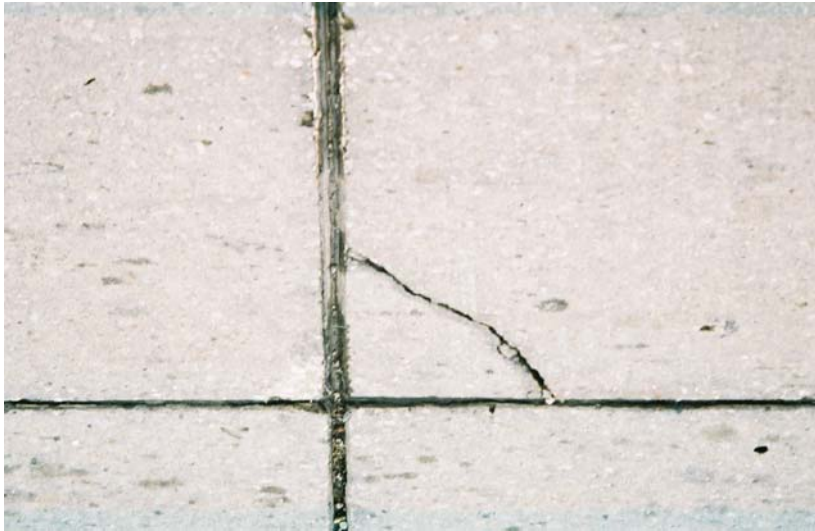
Figure 11a. Corner Cracking (Slight)
