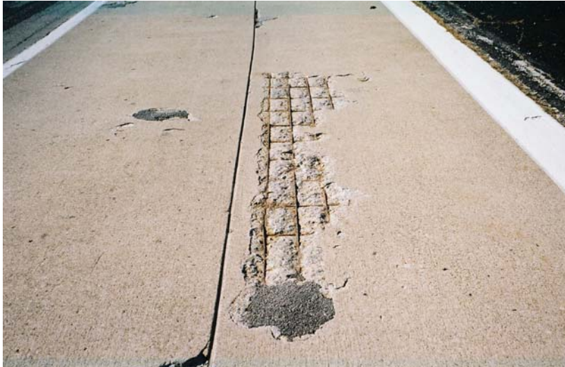
Figure 18a. Spall (Slight)
