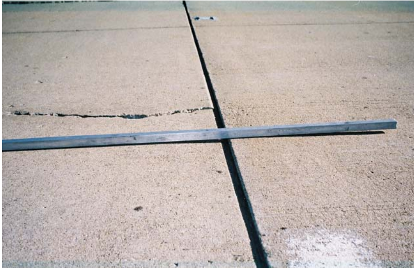
Figure 15a. Longitudinal Faulting (Slight)
