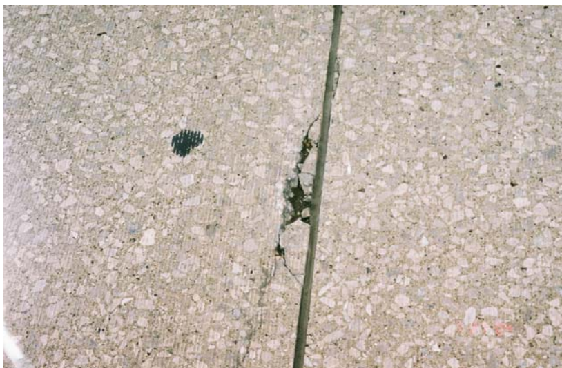
Figure 14c. D Cracking (Severe)
