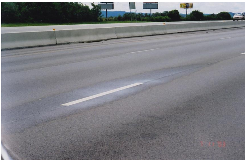
Figure 9c. Water Pumping (Severe)
