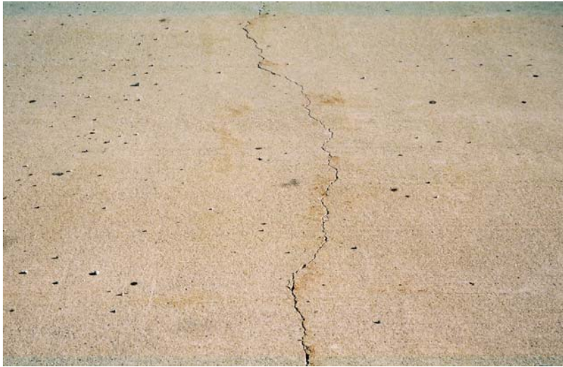
Figure 12a. Transverse Crack (Slight)
