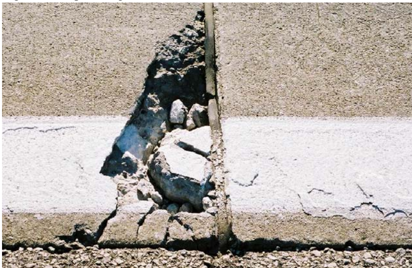
Figure 18b. Spall (Moderate)
