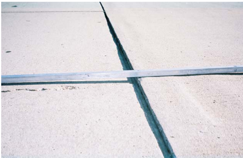
Figure 15b. Longitudinal Faulting (Moderate)
