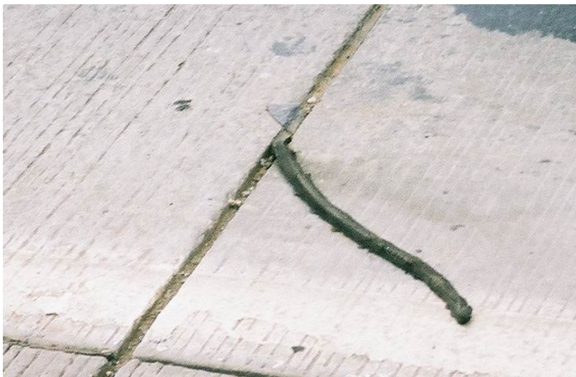
Figure 18c. Joint Seal Failure (Severe)
