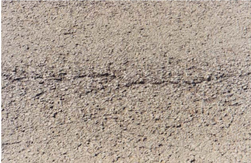
Figure 1a. Longitudinal Cracking (Slight)
