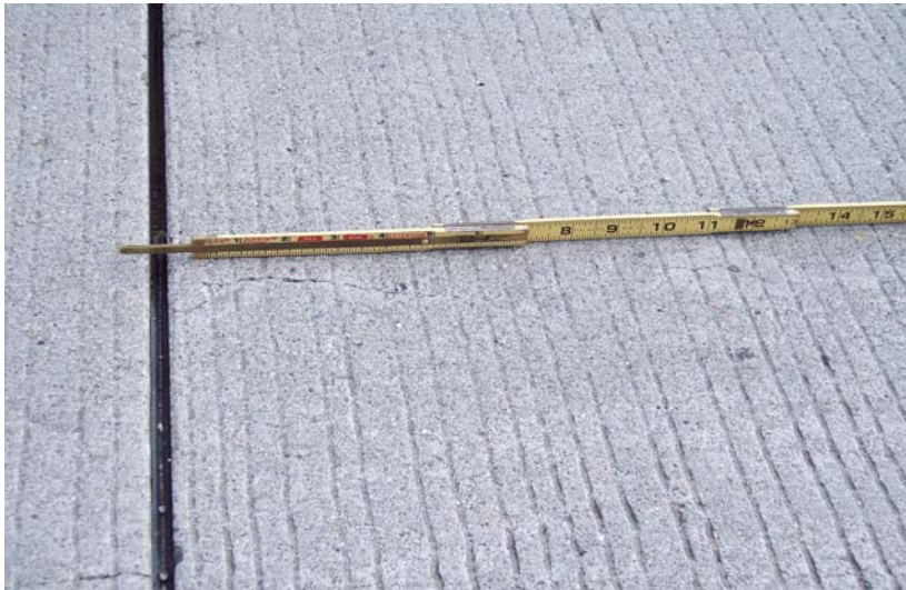
Figure 13a. Longitudinal Crack (Slight)
