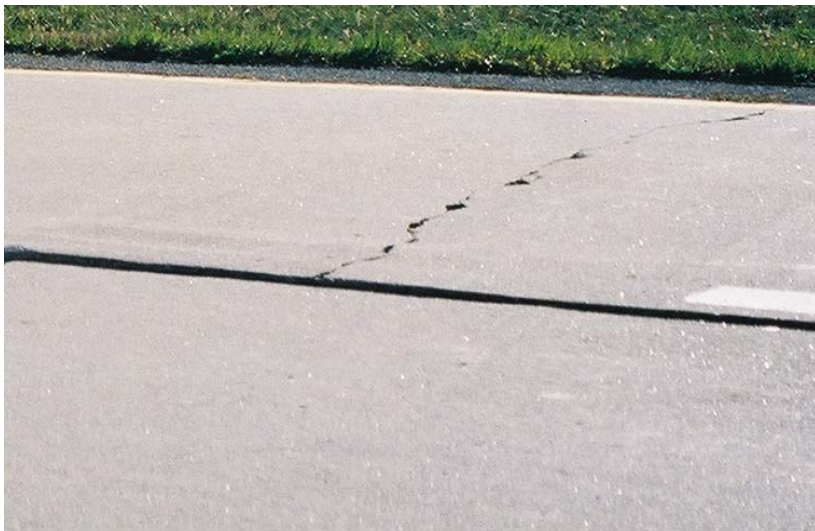
Figure 12b. Transverse Crack (Moderate)
