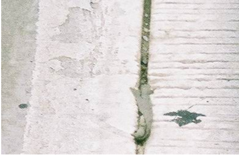
Figure 18 a. Joint Seal Failure (Slight)
