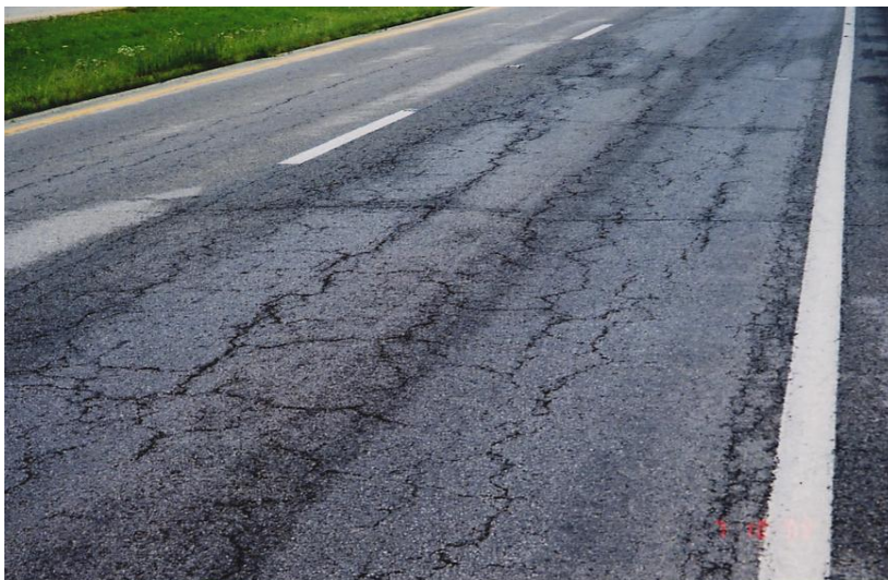
Figure 4c. Block Cracking (Severe)
