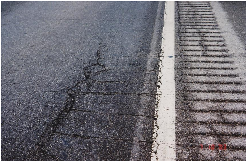
Figure 4b. Block Cracking (Moderate)
