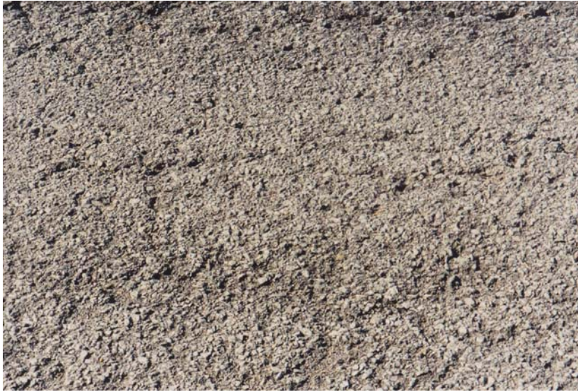
Figure 8a. Raveling (Slight)
