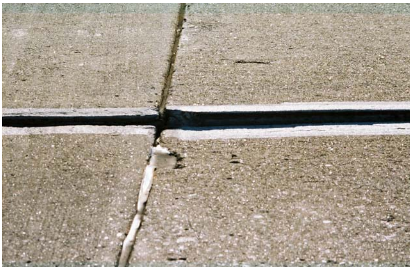
Figure 15c. Longitudinal Faulting (Severe)
