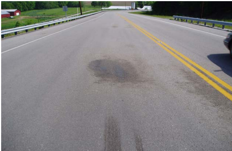
Figure 9b. Water Pumping (Moderate)
