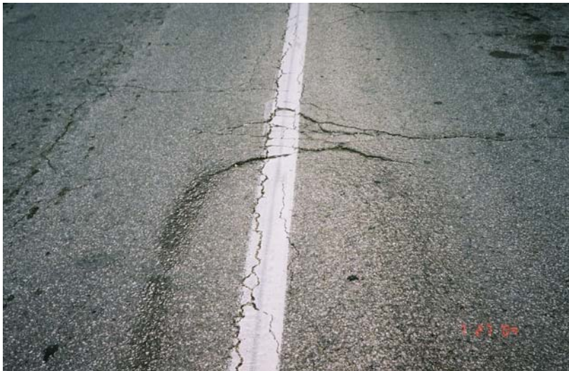
Figure 7a. Shoving (Slight)
