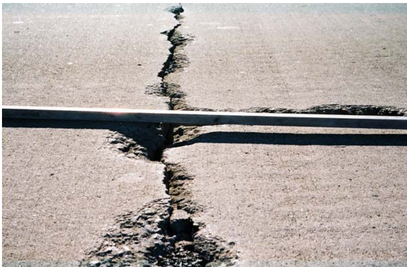
Figure 16b. Transverse Faulting (Moderate)
