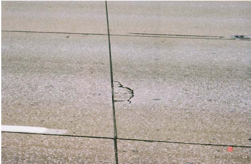
Figure 14b. D Cracking (Moderate)
