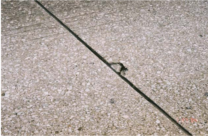
Figure 14a. D Cracking (Slight)
