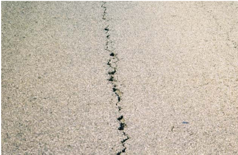
Figure 1b. Longitudinal Cracking (Moderate)
