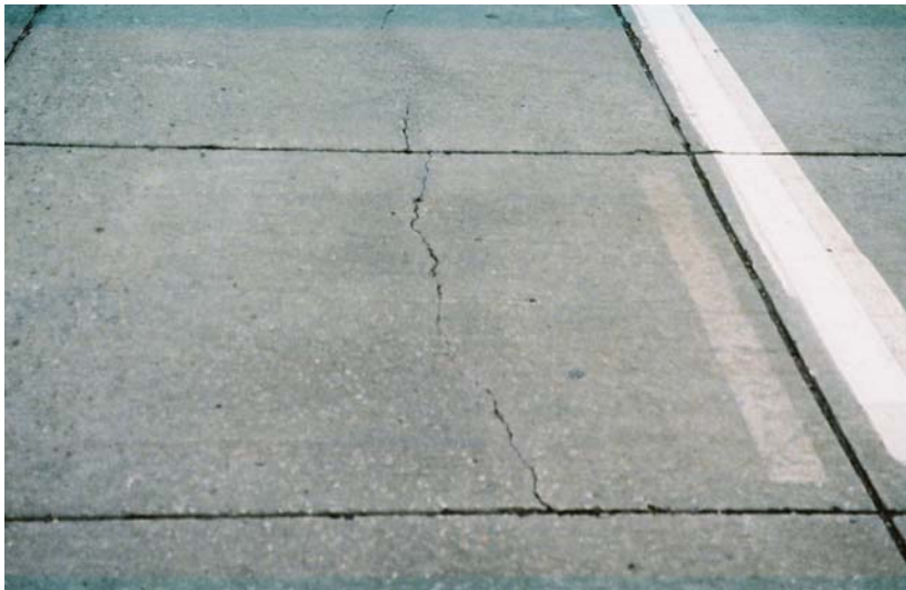
Figure 13a. Longitudinal Crack (Moderate)
