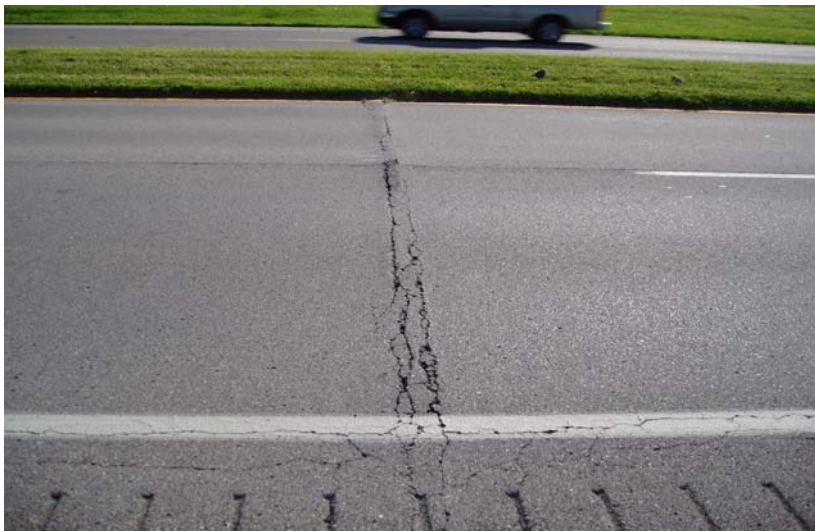
Figure 5b. Reflective Cracking (Moderate).
