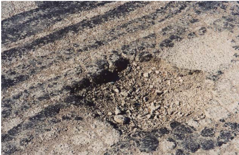
Figure 10b. Pothole (Moderate)
