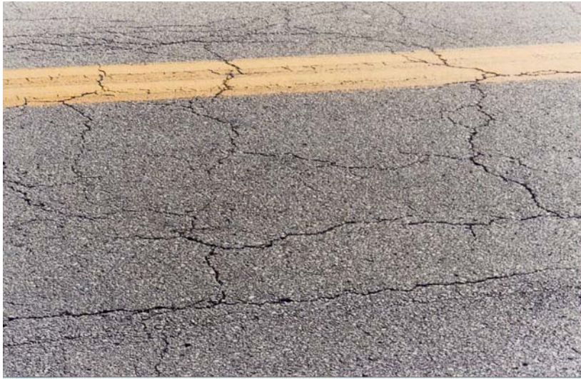
Figure 4a. Block Cracking (Slight)
