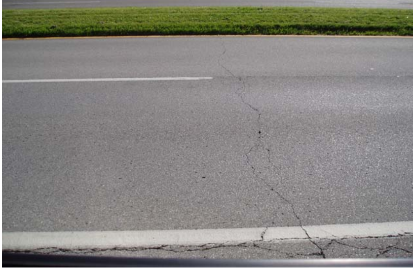
Figure 5a. Reflective Cracking (Slight).
