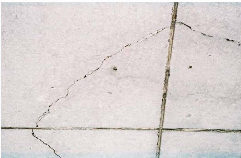
Figure 11c. Corner Crack (Severe)
