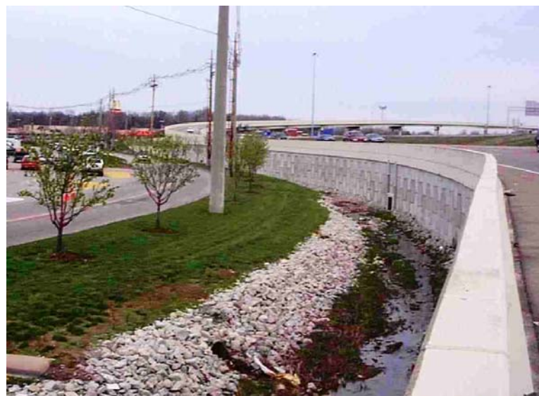
Figure 4. MSE Wall Tested in Jefferson County, ramp from US 60 to I 264 at St. Mathews Mall.
