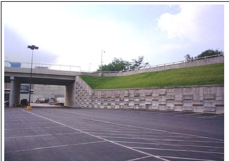
Figure 1. MSE Wall Tested in Fayette County; Parking Lot of Lexington Civic Center, below KY 1681.
