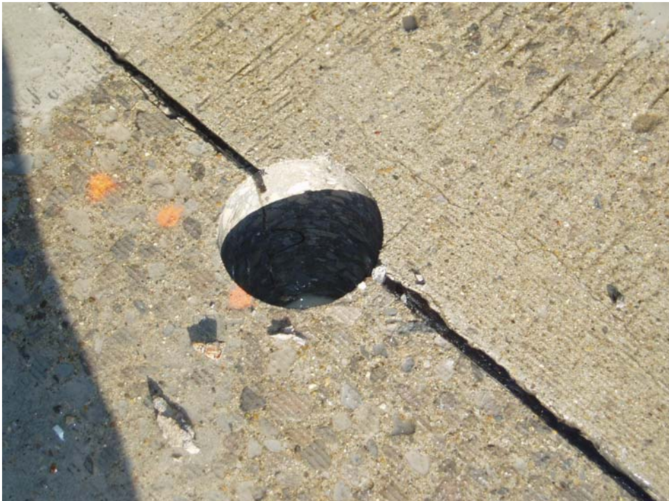
Figure 3. No Presence of Differential Settlement between Middle and inside Lane
