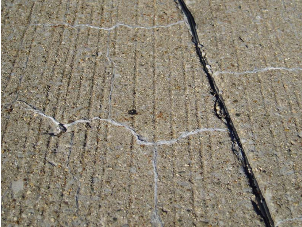
Figure 14: Hairline Cracking Around Concrete Joint
