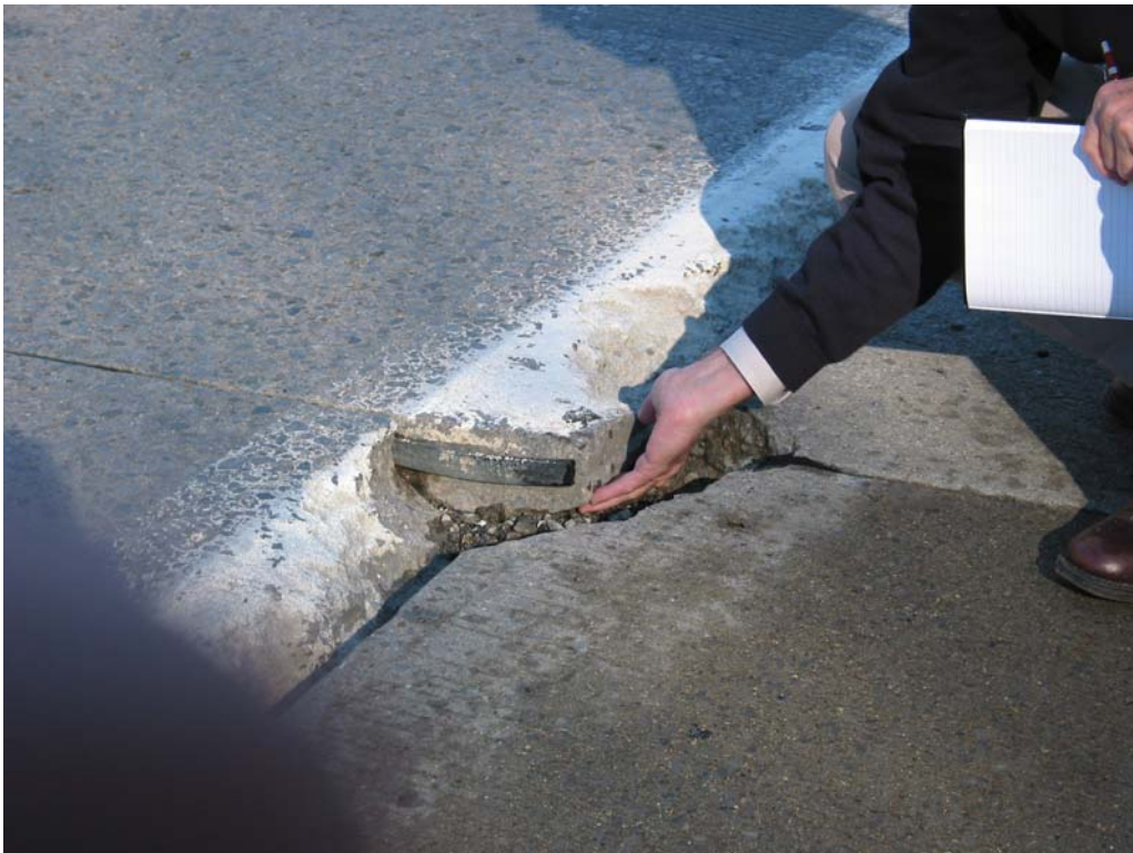
Figure 15: Depth of Spalled Joint
