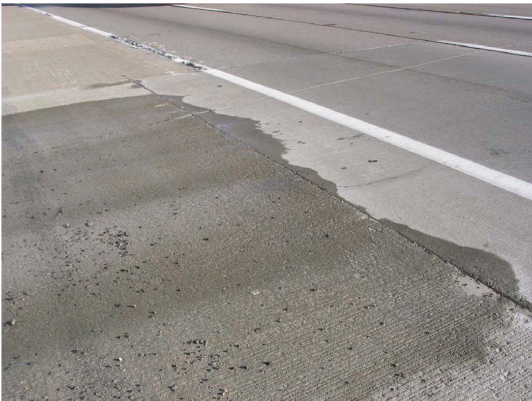
Figure 6: Water Bleeding Out of Shoulder Joint in Patched Area
