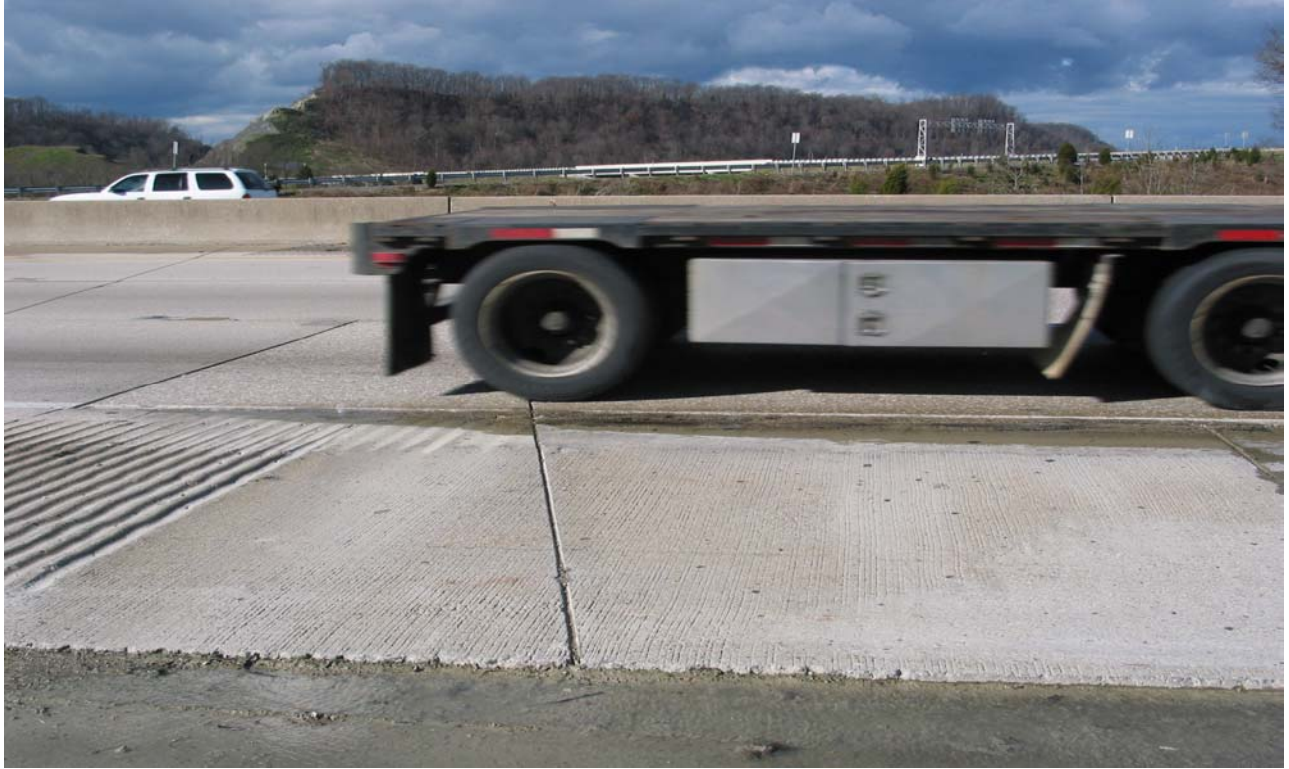
Figure 5: Water pumping Up from Shoulder Joint (Northbound)
