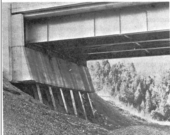
Figure 6. Views of western embankment slope failure and exposed abutment piling on the Bluegrass Parkway across Chaplin River (after Hopkins 1973).
