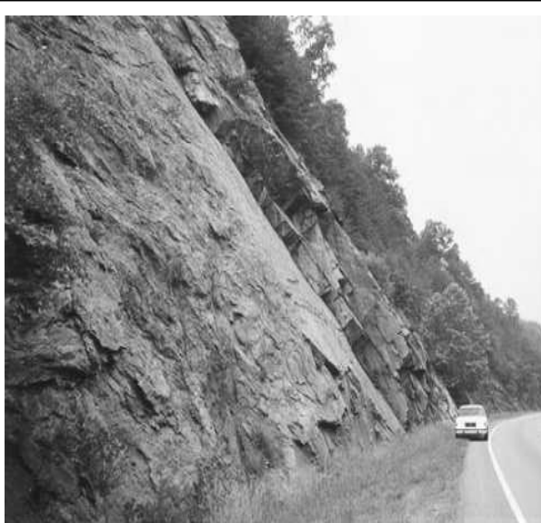
Figure 61. Another example of continuous joints and an adverse condition—tilted layers.
