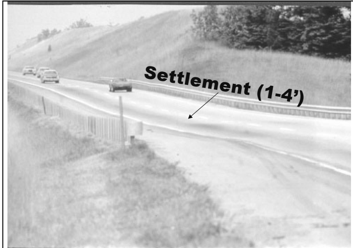
Figure 3. Example of large embankment settlement on I 75 about two decades after construction in Northern Kentucky (After Hopkins and Beckham, 1997, 1998).
