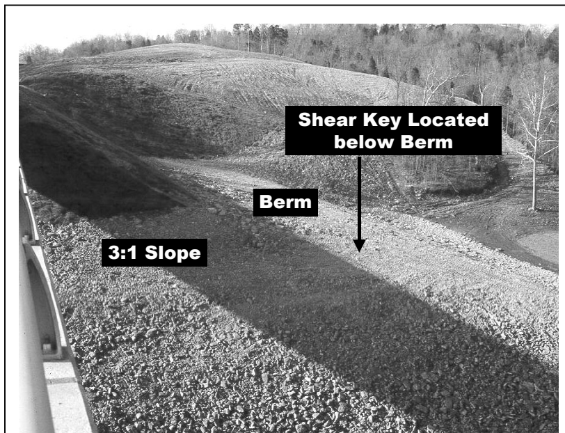
Figure 8. View of the construction of a shear key and berm to halt movement of the failing southern bridge approach embankment on U.S. 68 across Licking River in Nicholas County, Kentucky.
