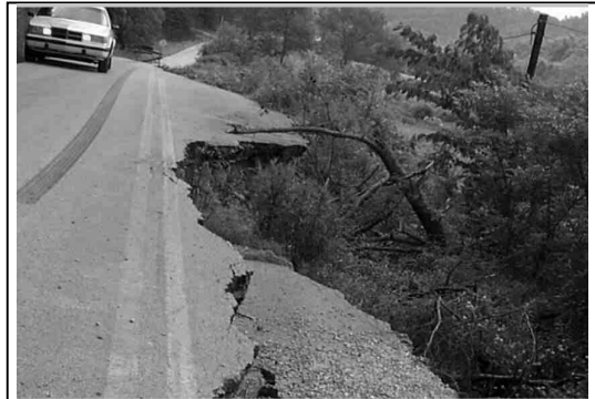
Figure 2. Highway embankment failure on KY 847 in Owsley County.
