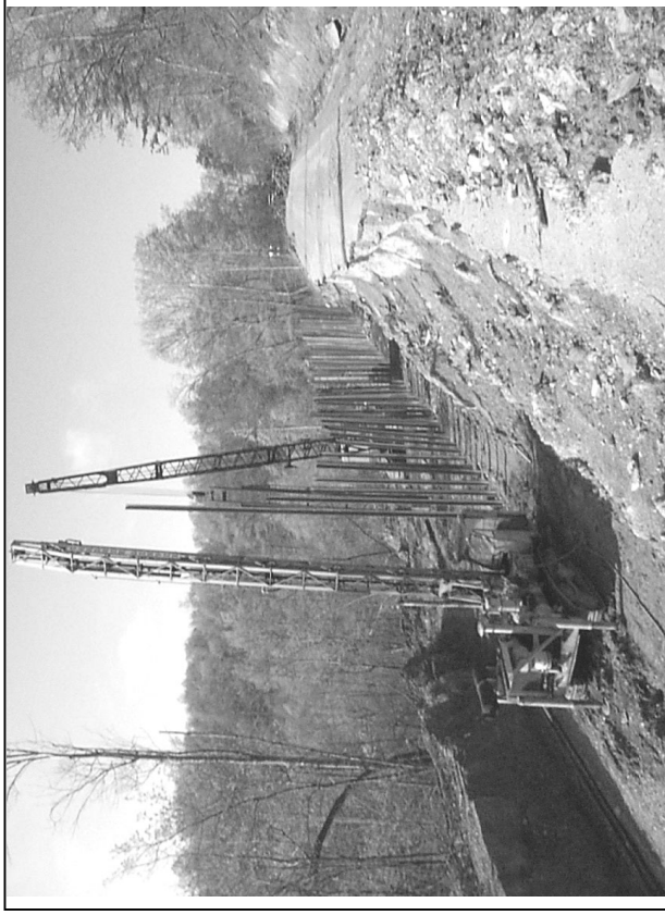
Figure 185. Installation in 1998 of railroad rails to form a wall to restrain a hillside landslide. Concrete panels were installed behind the anchored rails. The wall was backfilled with lightweight backfill, which consisted of cinders and shredded rubber tires (After Hopkins, Beckham, Sun, and Butcher 2002).
