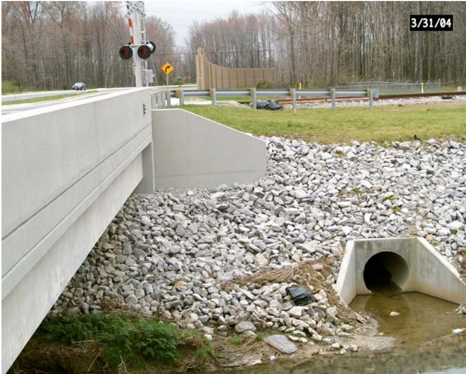
Figure 4. The rip rap and drains along the bank of Northern Ditch are shown adjacent to the Jefferson Boulevard bridge.
