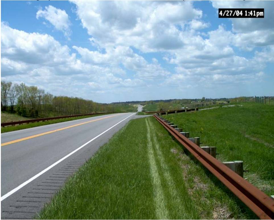
Figure 2. This is a Westward view along U.S. 150 toward the West end of the project. Note the use of grass shoulders and weathering steel guardrails.
