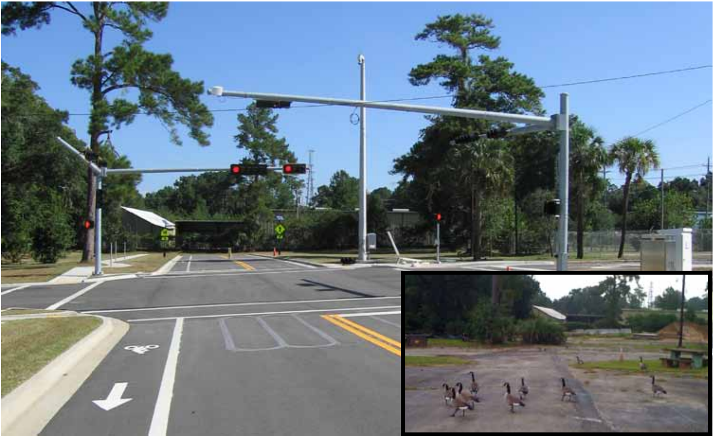
Researchers test a variety of traffic control devices at TERL’s new mast arm test intersection. Devices being tested include mast arm and pole-mounted traffic signals, traffic control cabinets, in-ground inductive-loop vehicle sensors, overhead vehicle sensors, closed circuit TV cameras, and pedestrian crosswalk signals. The intersection also features sidewalks, curbs, and bike lanes.
