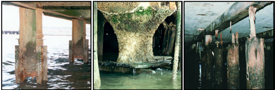
a) Corroded steel piles b) Degraded concrete pile c) Deteriorated timber piles
