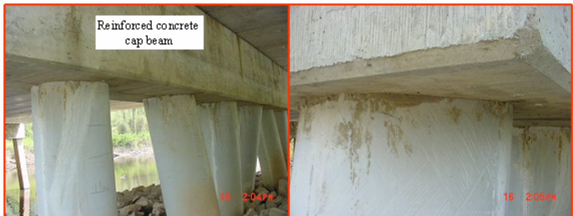
Figure 103. Photos. Pier No. 2 including the composite piles and reinforced concrete cap beam.
