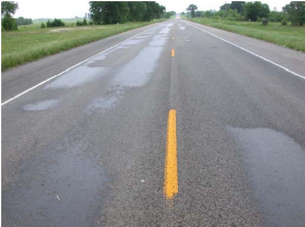
Figure 2-3 Flushed pavement (Lawson et al. 2007)
