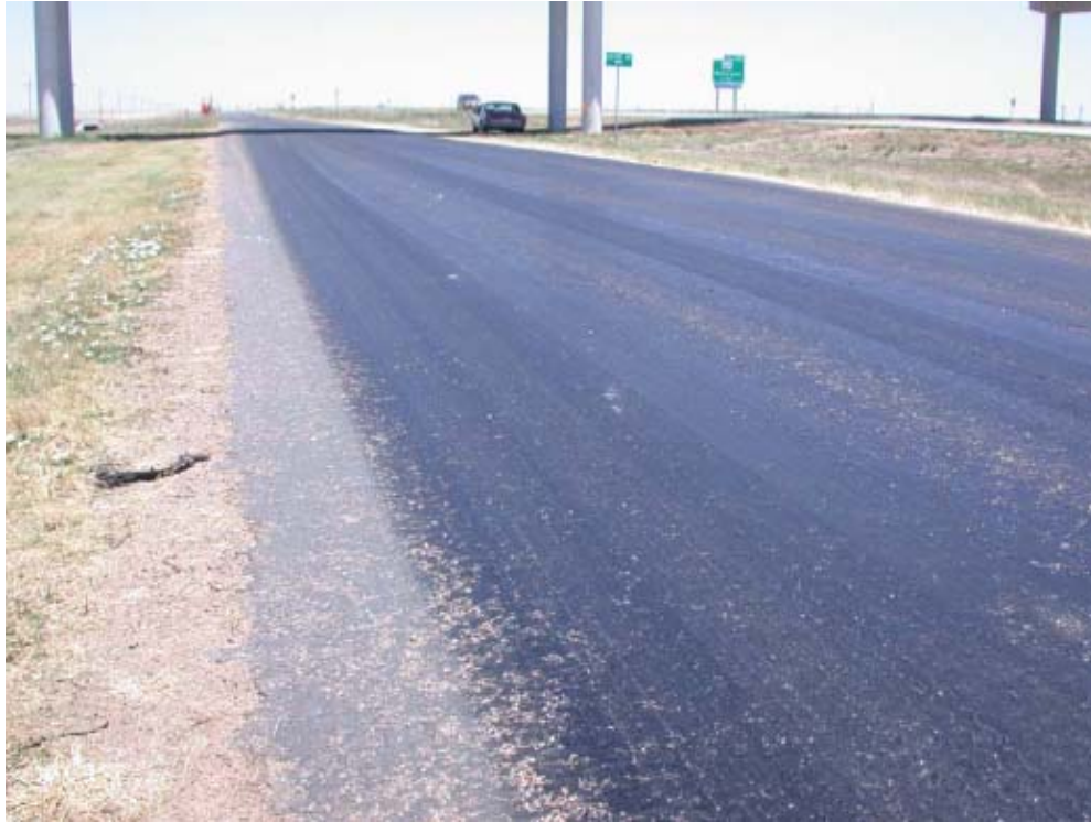
Figure 2-2 Bleeding due to heavy truck traffic and hot weather (Lawson et al. 2007)
