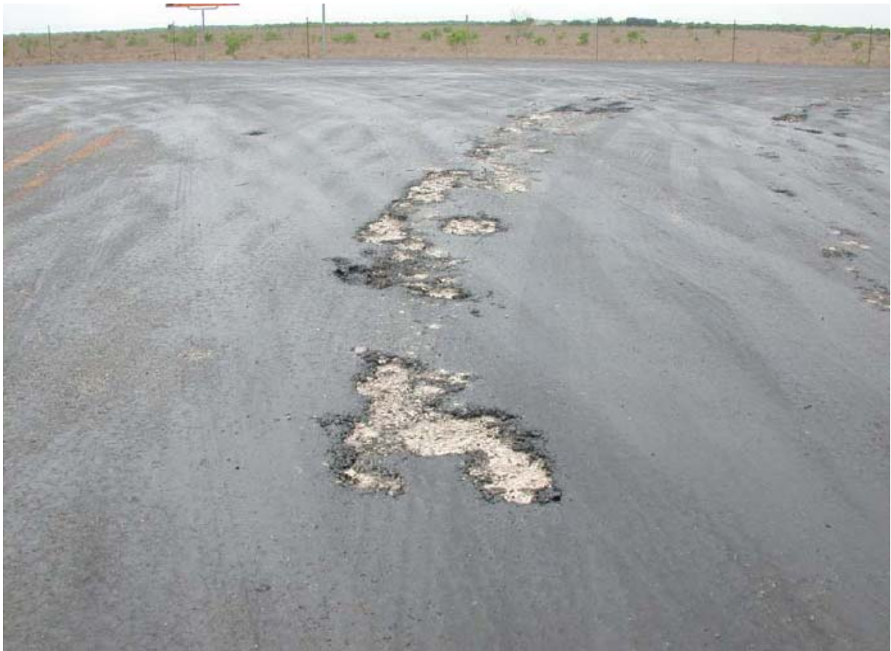
Figure 5-3 Chip seal damage caused by bleeding (Lawson et al. 2007)
