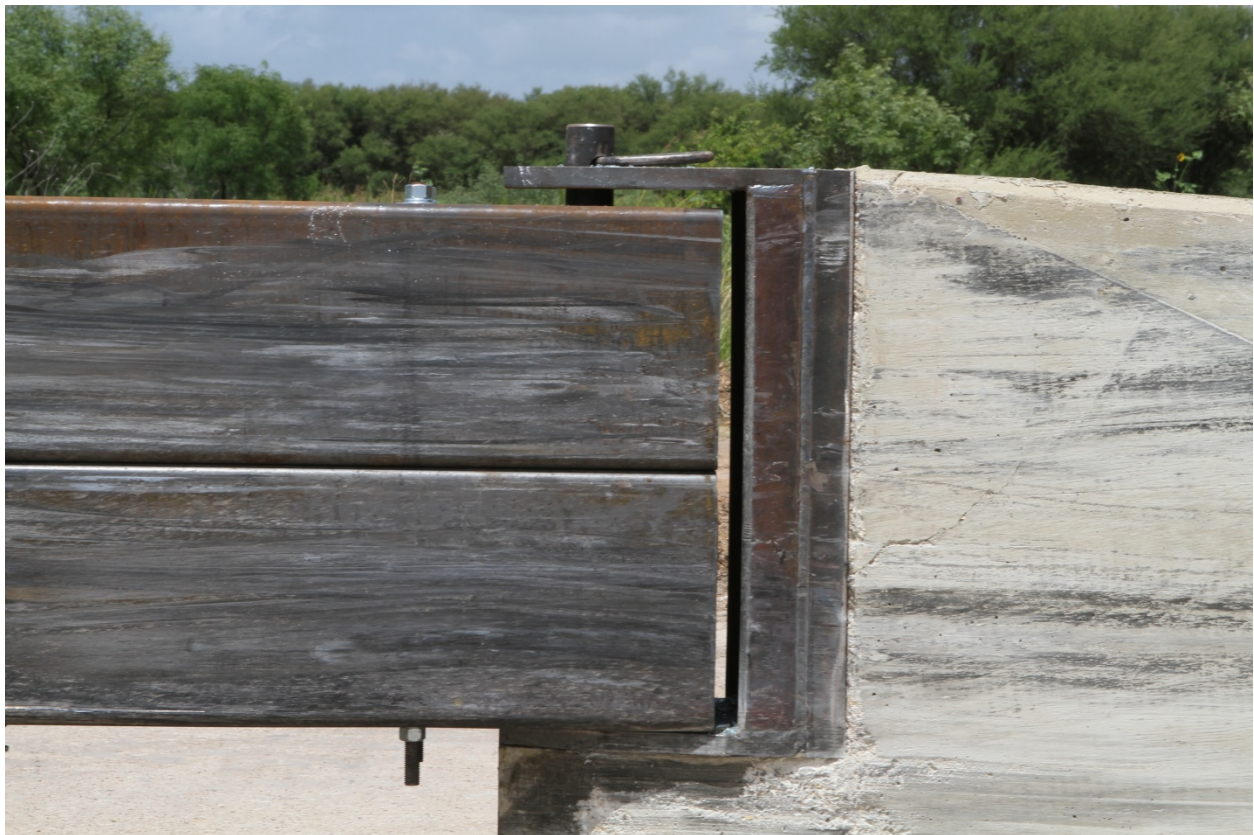
Figure 6.4. TxDOT Median Barrier Gate after Test No. 420020-6.
